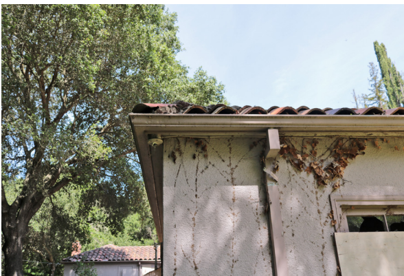
Remains of ivy growth along the south elevation (ARG, 2019).
