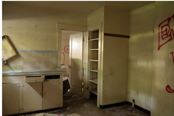
Note the missing door at the pantry of the West Kitchen (ARG, 2019).
