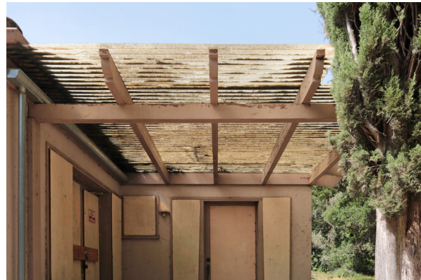
Corrugated plastic roof at pergola (ARG, 2019).
