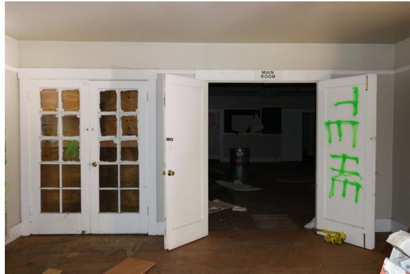
Graffiti at the original paneled wood door of the Entry (ARG, 2019).
