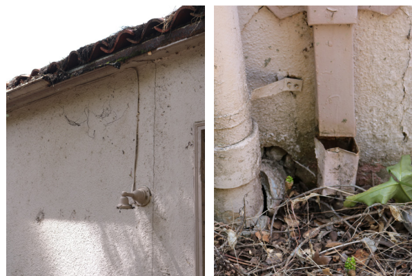
Missing segment of roof gutter (left); damaged rain leader (right); (ARG, 2019).
