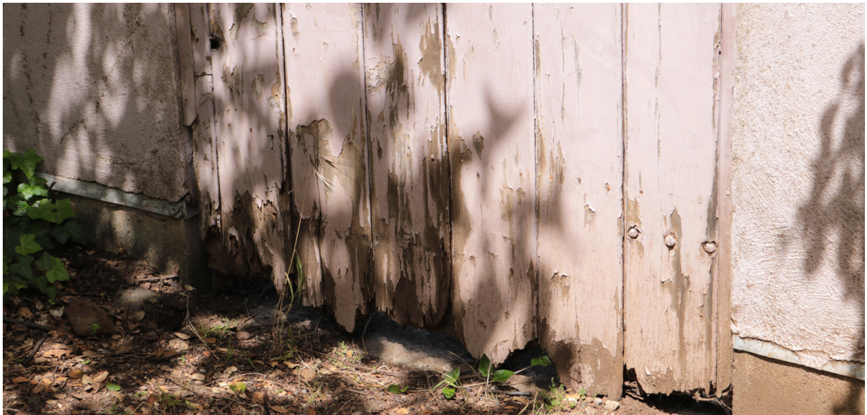
Detail view of wood deterioration at courtyard gate.
