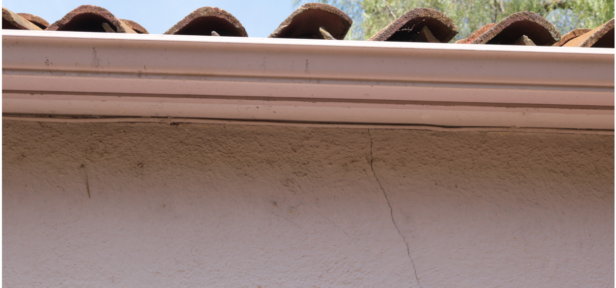
Detail view of stucco crack at south elevation.
