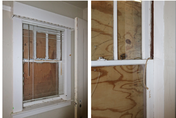
Typical original double-hung window in the Animal Room (left); damaged sash cord at Entry (right); (ARG, 2019).
