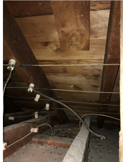
Photo #12: Roof Framing and Ceiling Joist at West Wing of the Building
