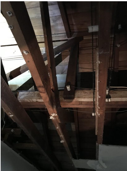
Photo #13: Roof Framing and Ridge Board at East Wing of the Building
