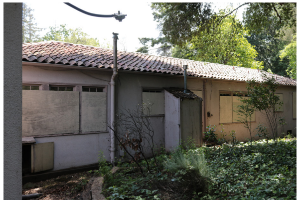
Plant growth along west elevation (ARG, 2019).
