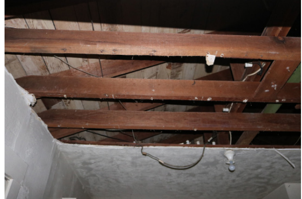
Missing drywall in the East Kitchen (ARG, 2019).
