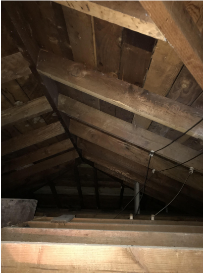
Photo #11: Roof Framing and Ridge Board at West Wing of the Building
