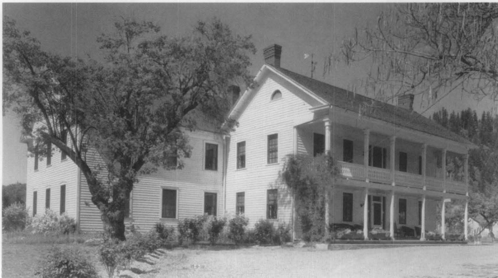
Figure 14. The treatment approach selected for a building usually is determined by the intended use of a property, funding prospects, and the findings of an investigation. The Wolf Creek Inn, operated by the Oregon Parks and Recreation Department, is among the most intact and oldest active travelers' inns in Oregon. The historic structure report outlined a rehabilitation treatment which included such work recommendations as repairs to specific historic fabric, landscape restoration and site improvements, and upgrading of the building's mechanical and electrical systems. Photo: Historic American Building Survey, 1934.
