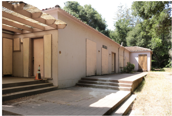
View of north elevation looking west. Note the lack of handrails at both sets of stairs (ARG, 2019).
