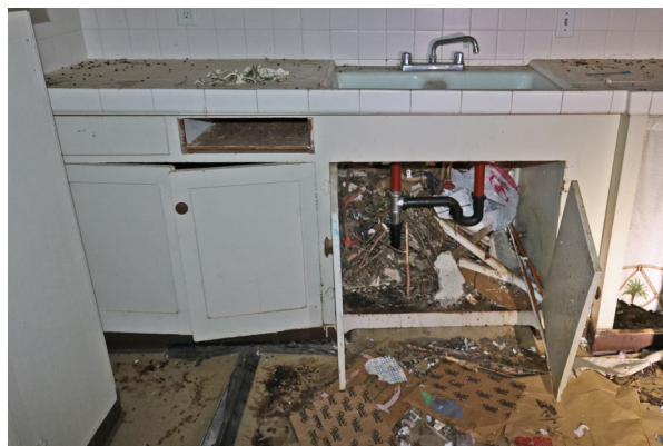
Large rodent nest at the sink base cabinet in the East Kitchen. Note the missing drawer and missing hardware (ARG, 2019).
