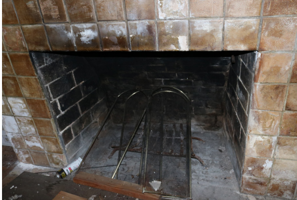
Firebox and ceramic tile surround at the fireplace in the Main Room (ARG, 2019).
