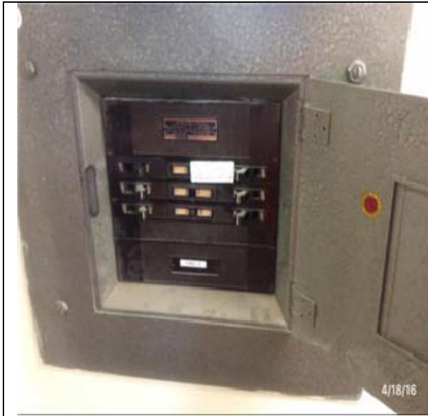
D5012 Low Tension Service & Dist:- View of Panelboard - 120/240volts, 100amp
