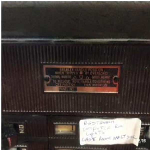
D5012 Low Tension Service & Dist:- View of Panelboard - 120/240volts, 100amp
