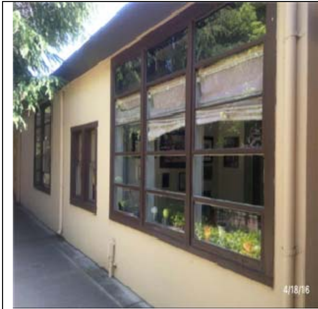
B2021 Windows:- View of Steel Window Units - Casement, Double Hung, Vent or Sliding
