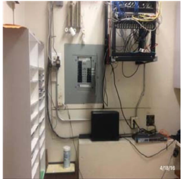
D5012 Low Tension Service & Dist:- View of Panelboard - 120/240volts, 60 to 2000amp
