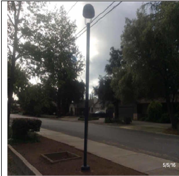
G4021 Fixtures & Transformers:- View of 20' High Site Lighting
