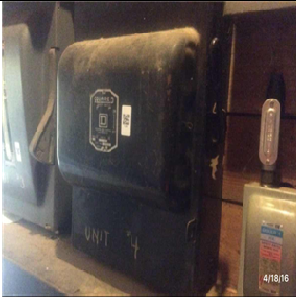
D5012 Low Tension Service & Dist:- View of Panelboard - 120/240volts, 200amp
