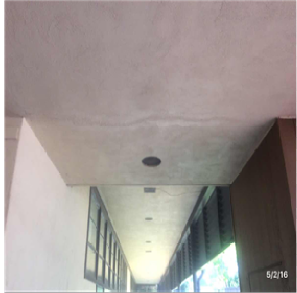
D5022 Lighting Equipment:- View of Recessed Can Light Fixtures
