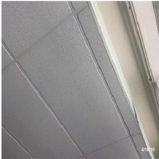
C3032 Suspended Ceilings:- View of Acoustic Ceiling System - Standard
