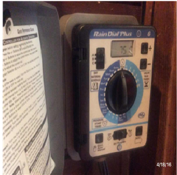
G2057 Irrigation Systems:- View of Complete Irrigation System
