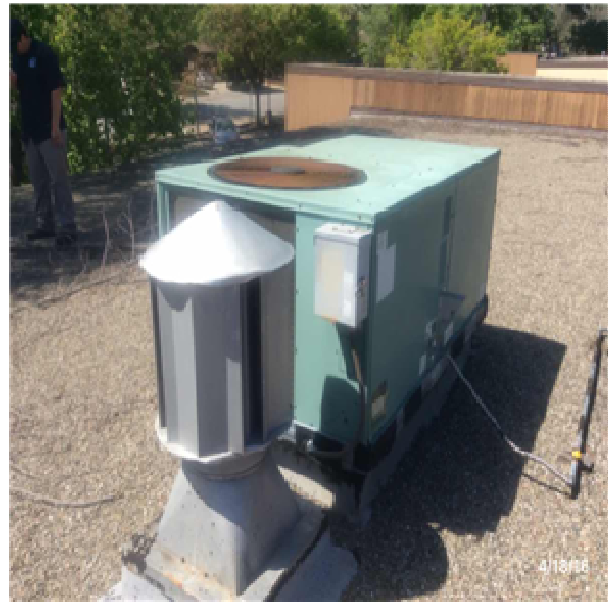
D3052 Package Units:- View of Packaged Outdoor - Cooling and Heating
