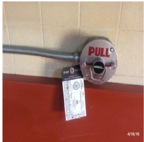
D4095 Hood & Duct Fire Protection:- View of Hood & Duct Fire Protection
