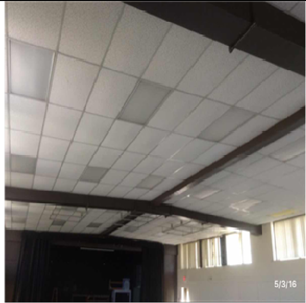
D5022 Lighting Equipment:- View of Fluor. Light 2' x 4' Recess/Surface Mounted Fixtures
