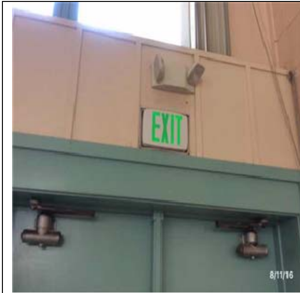
D5092 Emergency Light & Power Systems:- View of Exit Lights L.E.D
