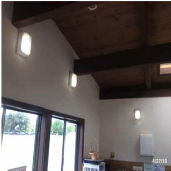
D5022 Lighting Equipment:- View of Incandescent Exterior Light Fixture(s)
