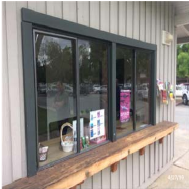
B2021 Windows:- View of Aluminum Window Units - Casement, Double Hung, Vent or Sliding
