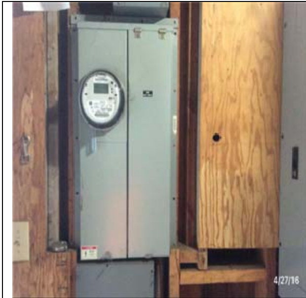
D5012 Low Tension Service & Dist:- View of Switchboard - 120/208volts, 400 to 2000amp
