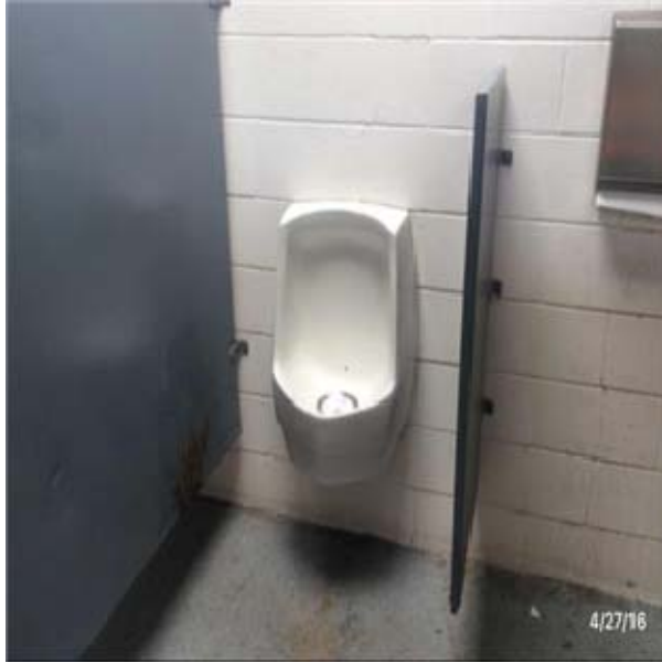
D2012 Urinals:- View of Wall Hung Urinal
