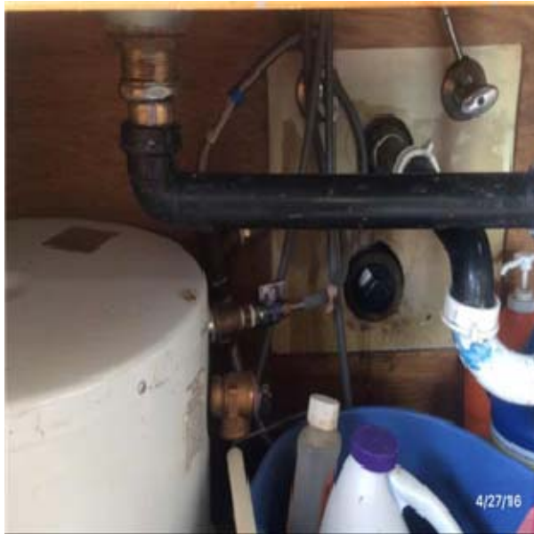
D2031 Waste Piping:- View of Sanitary Water Gravity Discharge
