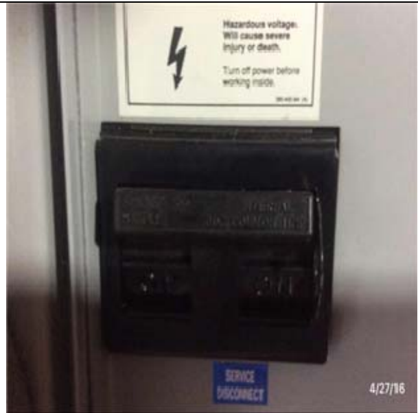
D5012 Low Tension Service & Dist:- View of Switchboard - 120/208volts, 400 to 2000amp
