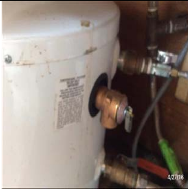
D2022 Hot Water Service:- View of Domestic Hot Water Heater - Electric
