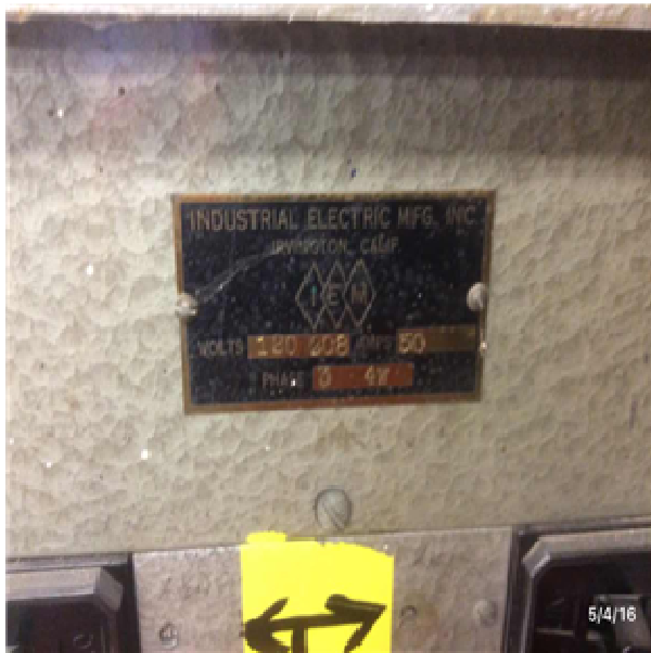
D5012 Low Tension Service & Dist:- View of Panelboards - 120/208volts, 60amp
