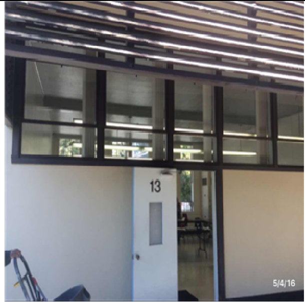
B2021 Windows:- View of Steel Window Units - Casement, Double Hung, Vent or Sliding
