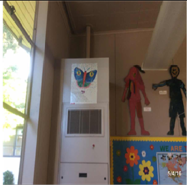
D3021 Boilers:- View of Furnace - Gas
