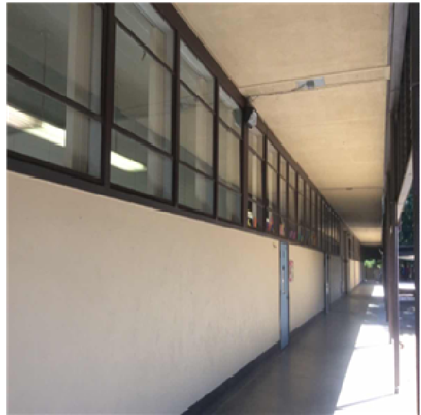
B2021 Windows:- View of Steel Window Units - Casement, Double Hung, Vent or Sliding
