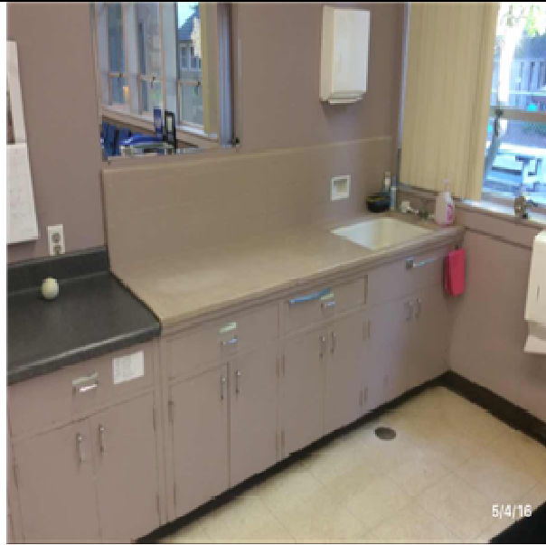
D2013 Lavatories:- View of Vanity Top Lavatories
