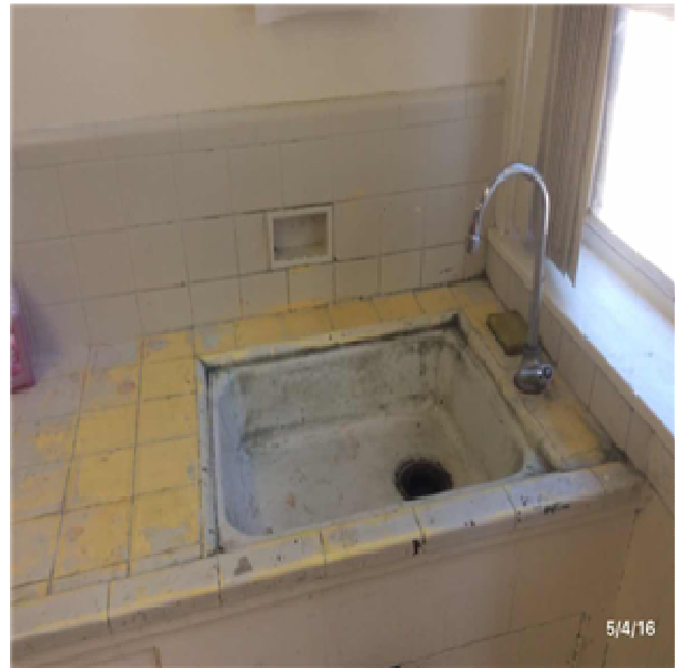
D2013 Lavatories:- View of Vanity Top Lavatories
