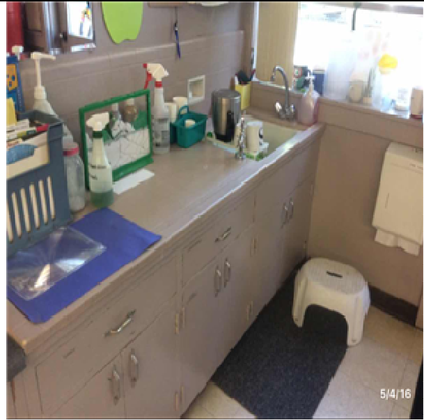
D2013 Lavatories:- View of Vanity Top Lavatories
