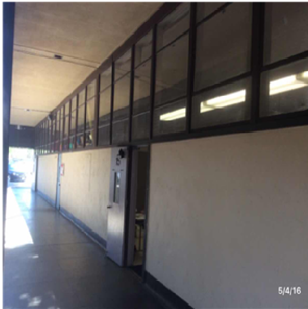
B2021 Windows:- View of Steel Window Units - Casement, Double Hung, Vent or Sliding
