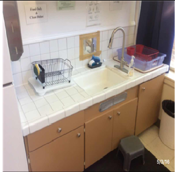
D2013 Lavatories:- View of Vanity Top Lavatories
