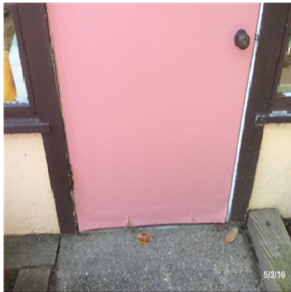
B2032 Solid Exterior Doors:- View of Exterior Single Solid Core Wood Doors
