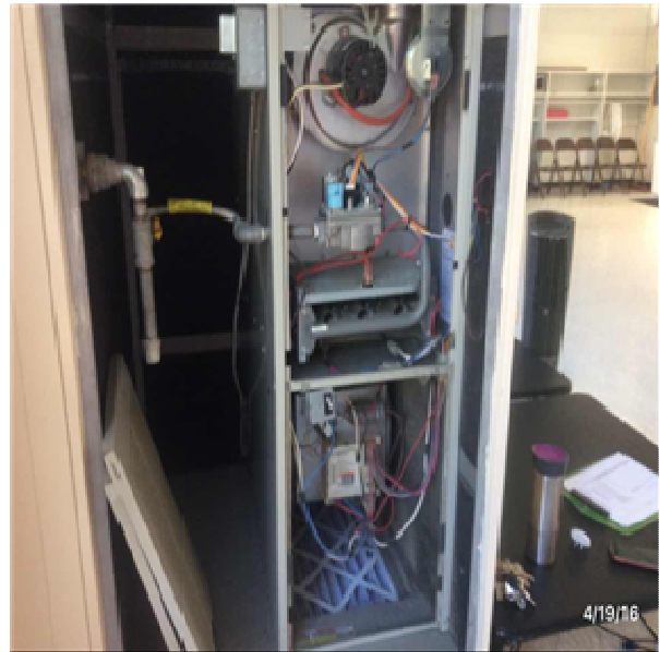
D3021 Boilers:- View of Furnace – Gas
