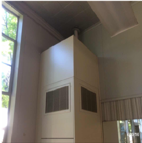
D3021 Boilers:- View of Furnace – Gas
