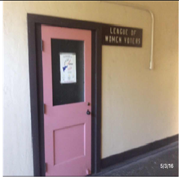
B2032 Solid Exterior Doors:- View of Exterior Single Solid Core Wood Doors
