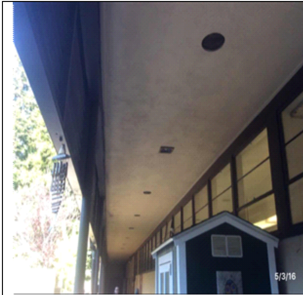
D5022 Lighting Equipment:- View of Recessed Can Light Fixture(s)
