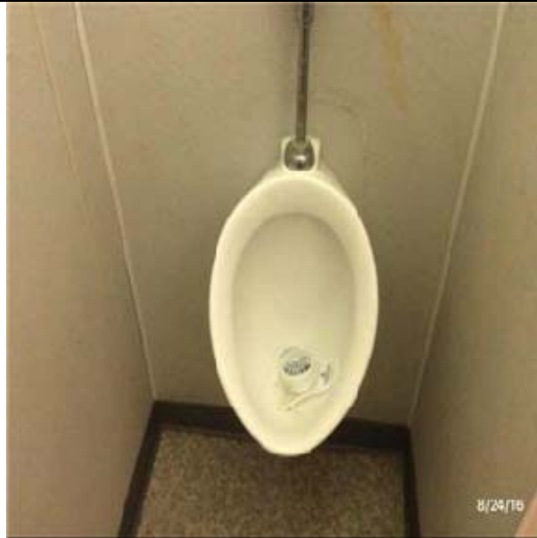
D2012 Urinals:- View of Wall Hung Urinals
