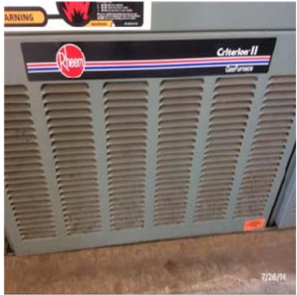
D3021 Boilers:- View of Furnace - Gas #2
