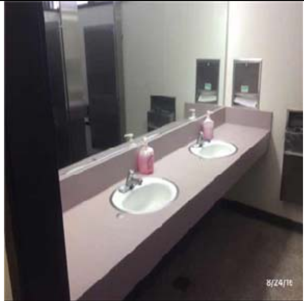
D2013 Lavatories:- View of Vanity Top Lavatories
