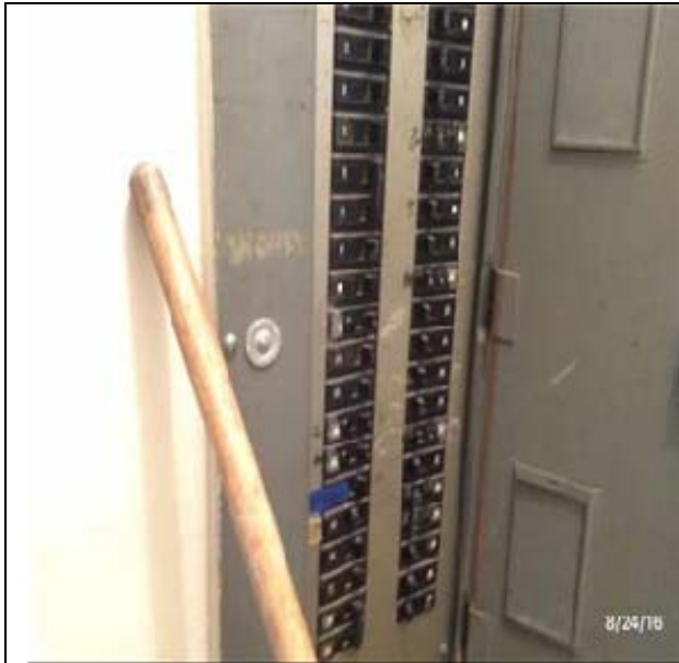
D5012 Low Tension Service & Dist:- View of Panelboard - 120/240volts, 200 to 1200amp
