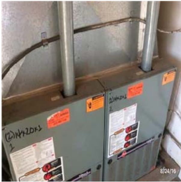
D3021 Boilers:- View of Furnace - Gas #1
