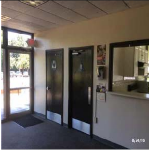
D5092 Emergency Light & Power Systems:- View of Exit Lights
