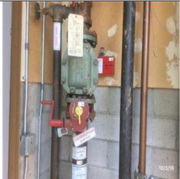
D4011 Sprinkler Water Supply:- View of Wet-Pipe Sprinkler System
