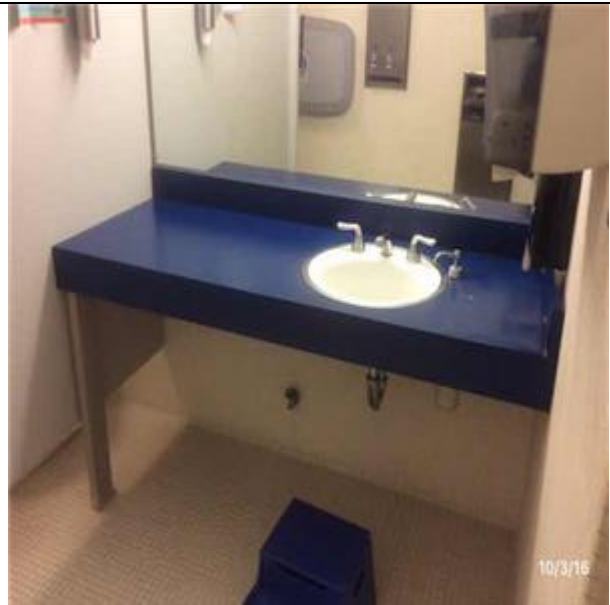
D2013 Lavatories:- View of Vanity Top Lavatories
