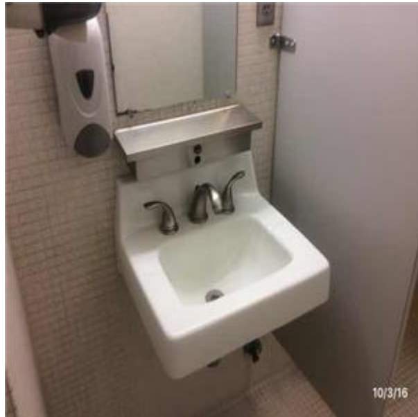
D2013 Lavatories:- View of Wall Hung Lavatories
