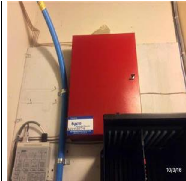
D5037 Fire Alarm Systems:- View of Fire Alarm System (Full System Inc. Panel)
