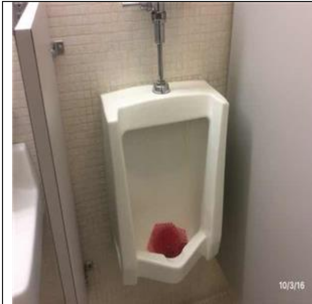
D2012 Urinals:- View of Wall Hung Urinals
