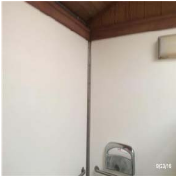
C3012 Wall Finishes to Interior Walls:- View of FRP Finish to Wall
