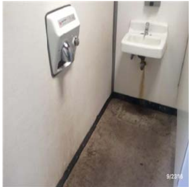
D2013 Lavatories:- View of Wall Hung Lavatories
