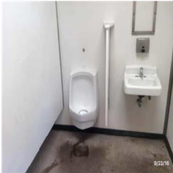
D2012 Urinals:- View of Wall Hung Urinal
