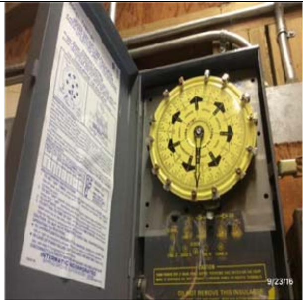
D5036 Clock and Program Systems:- View of Time Clock
