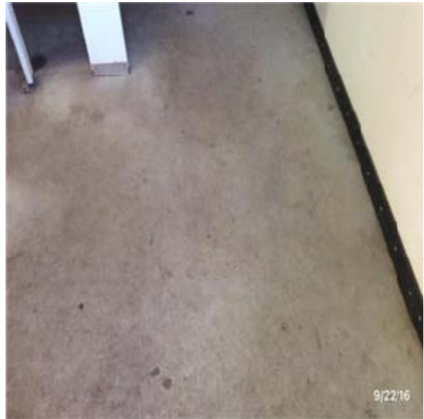
C3023 Hardeners and Sealers:- View of Floor Paint - Non Slip
