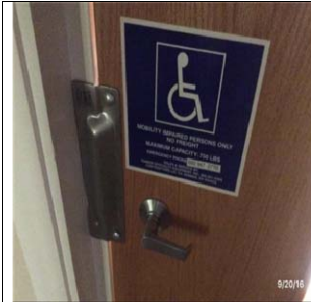
D1094 Conveyors:- View of ADA - Wheelchair lift two levels
