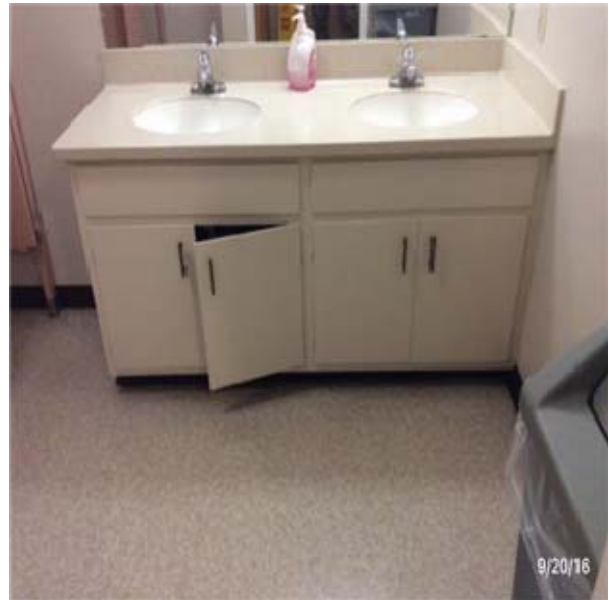
D2013 Lavatories:- View of Vanity Top Lavatories
