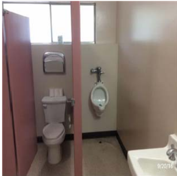
D2012 Urinals:- View of Wall Hung Urinals
