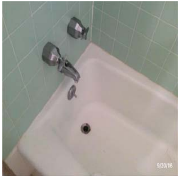
D2015 Bathtubs:- View of Bathtub
