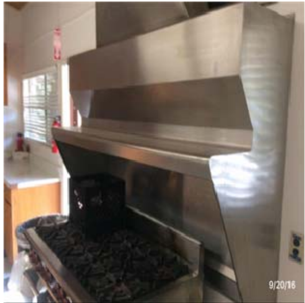
D3042 Exhaust Ventilation Systems:- View of Fume Hood Exhaust System - Standard
