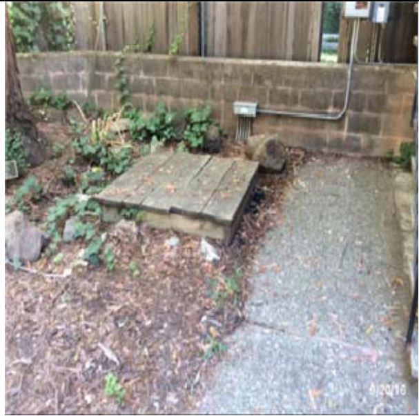
D2031 Waste Piping:- View of Basement/Foundation drainage sump pump
