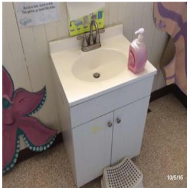
D2013 Lavatories:- View of Vanity Top Lavatories
