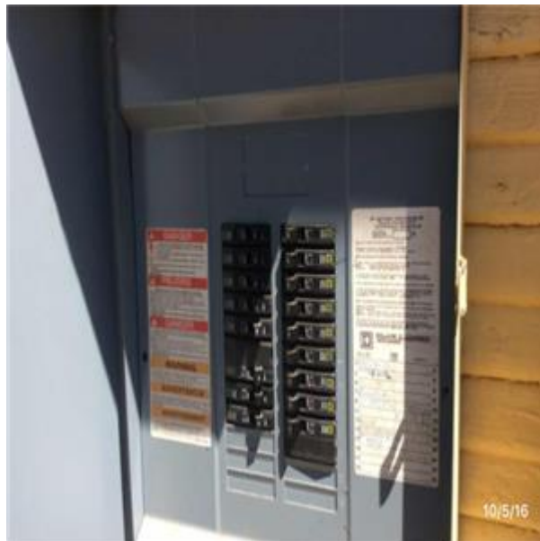
D5012 Low Tension Service & Dist:- View of Panelboard - 120/208volts, 60 to 2000amp
