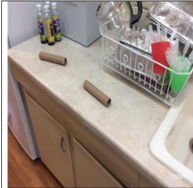
E2012 Fixed Casework:- View of Counter Top
