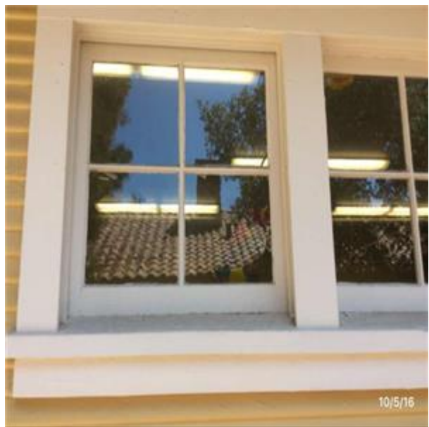
B2021 Windows:- View of Wood Window Units - Casement, Double Hung, Vent or Sliding
