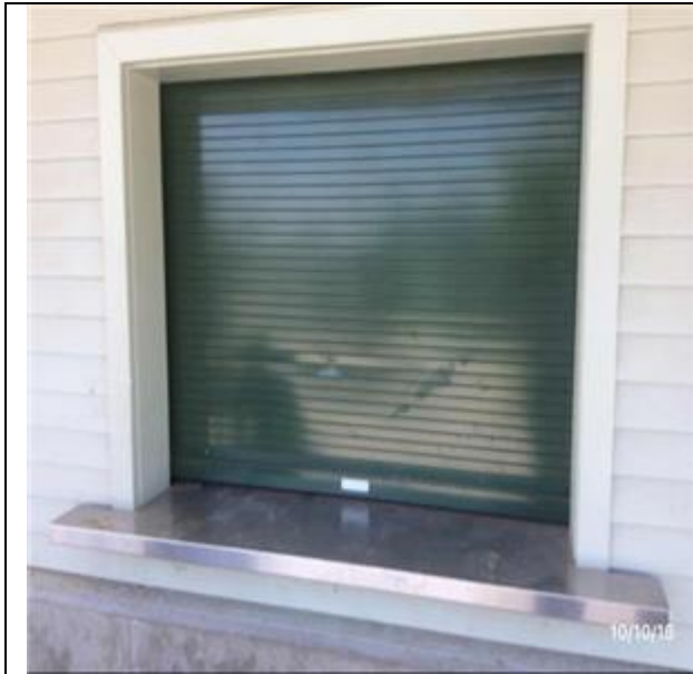
B2034 Overhead Doors:- View of Rolling Overhead Door to Counter
