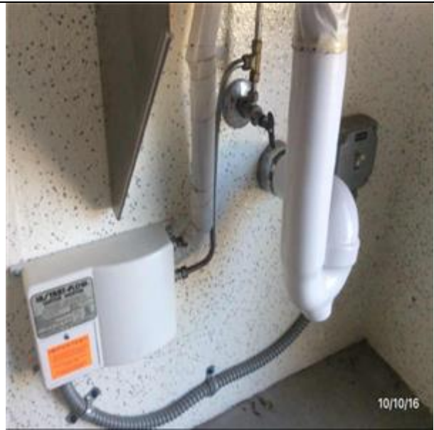
D2022 Hot Water Service:- View of Insta-Hot under Counter Water Heater
