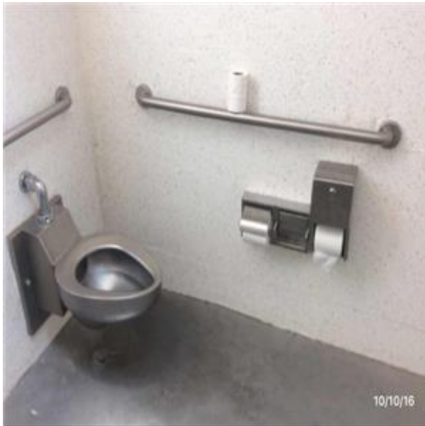
D2011 Water Closets:- View of Wall Mounted Water Closets - Stainless Steel
