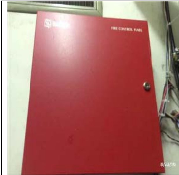
D5037 Fire Alarm Systems:- View of Fire Alarm System (Full System Inc. Panel)
