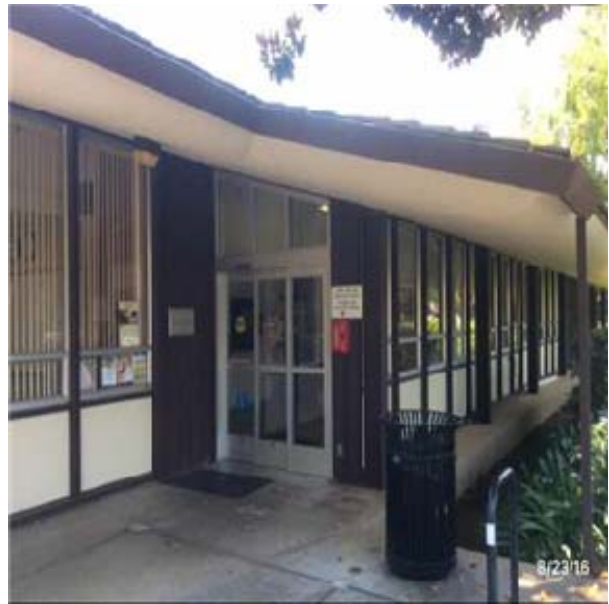
B2031 Glazed Doors & Entrances:- View of Storefronts - Glazed Aluminum Framed with Sliding Door Panels
