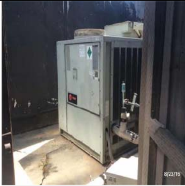
D3031 Chilled Water Systems:- View of Air Cooled Water Chiller Unit - Outdoor Unit
