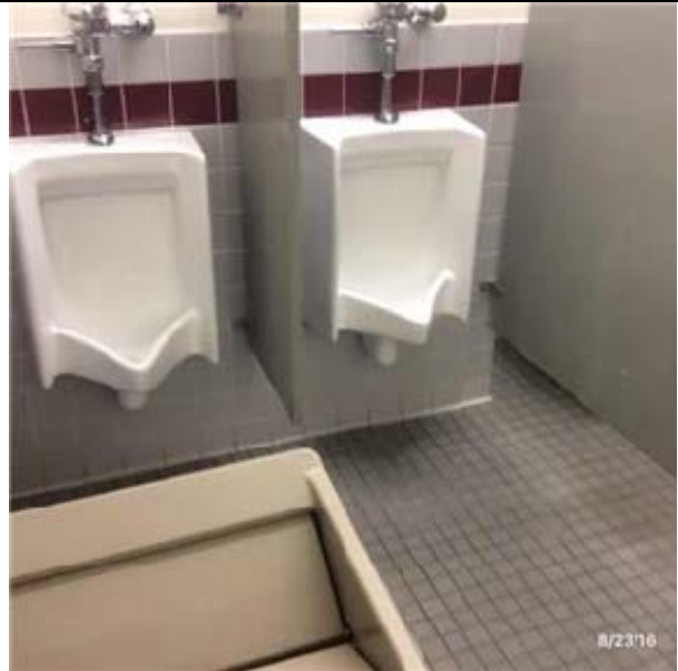
D2012 Urinals:- View of Wall Hung Urinals
