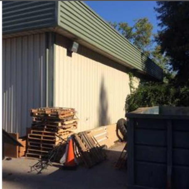
B2011 Exterior Wall Construction:- View of Cladding - Prefomed Corrugated Metal Wall Panels
