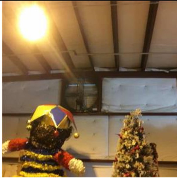
D3042 Exhaust Ventilation Systems:- View of Exhaust Fan - Wall Mounted
