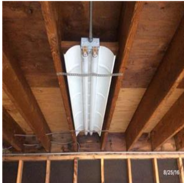
D5022 Lighting Equipment:- View of Fluorescent Light Fixtures
