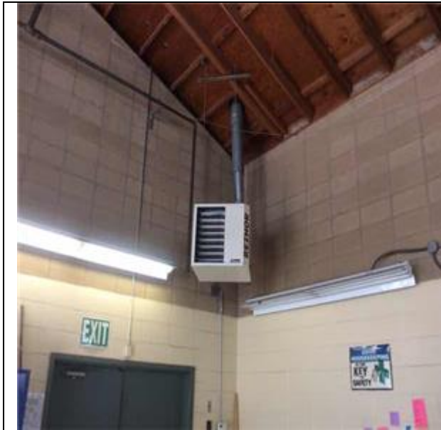
D3051 Terminal Self-Contained Units:- View of Unit Heater - Gas Fired Suspended - 100 MBH
