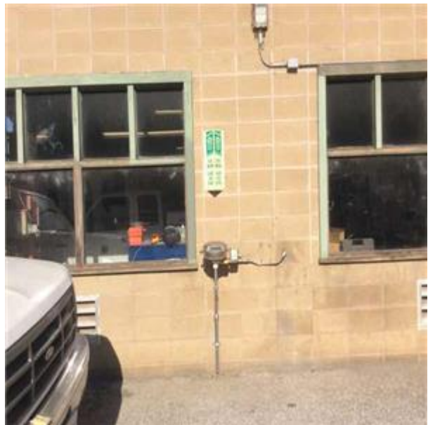
D2016 Wash Fountains:- View of Emergency Eye Wash
