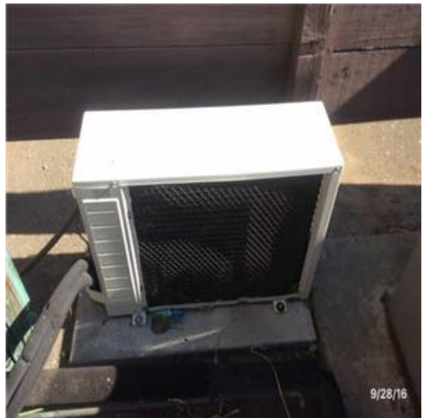
D3032 Direct Expansion Systems:- View of Split-System (Outdoor and Indoor Unit)
