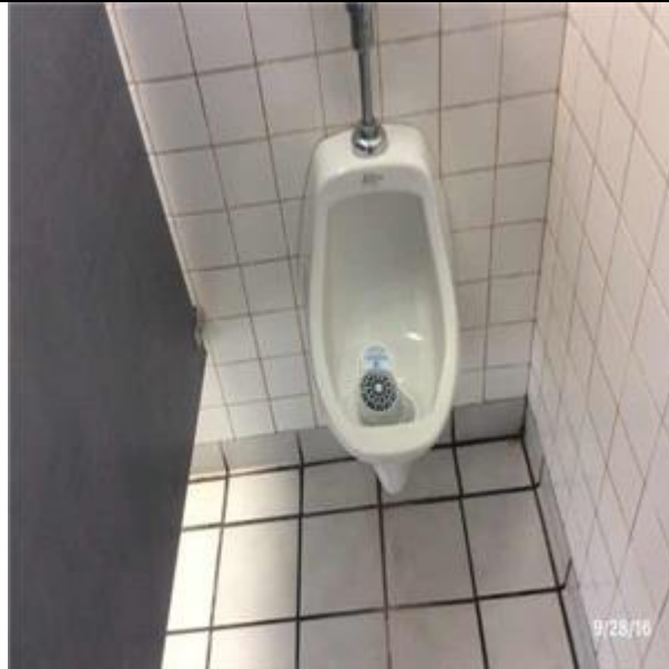
D2012 Urinals:- View of Wall Hung Urinals
