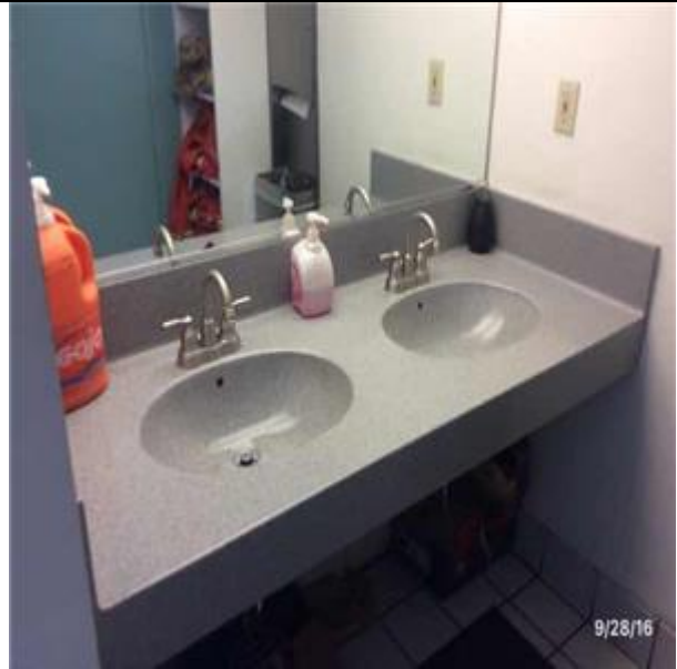
D2013 Lavatories:- View of Vanity Top Lavatories
