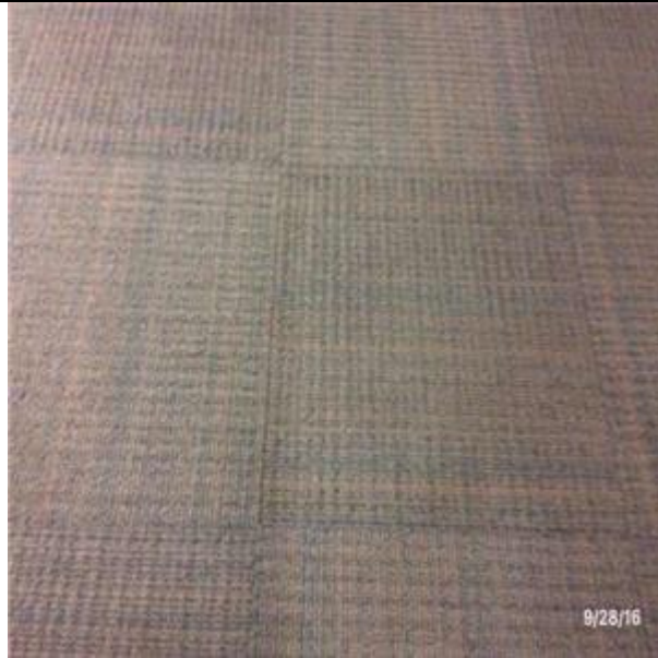
C3025 Carpeting:- View of Carpet Tiles – Standard
