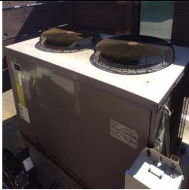
D3032 Direct Expansion Systems:- View of Split-System (Outdoor Unit Only - Compressor and Condenser)
