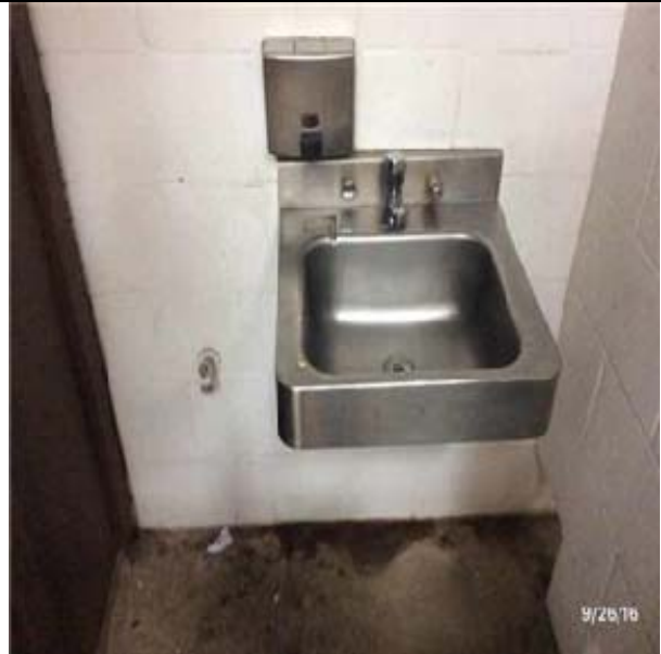
D2013 Lavatories:- View of Wall Hung Lavatories
