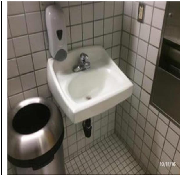
D2013 Lavatories:- View of Wall Hung Lavatories
