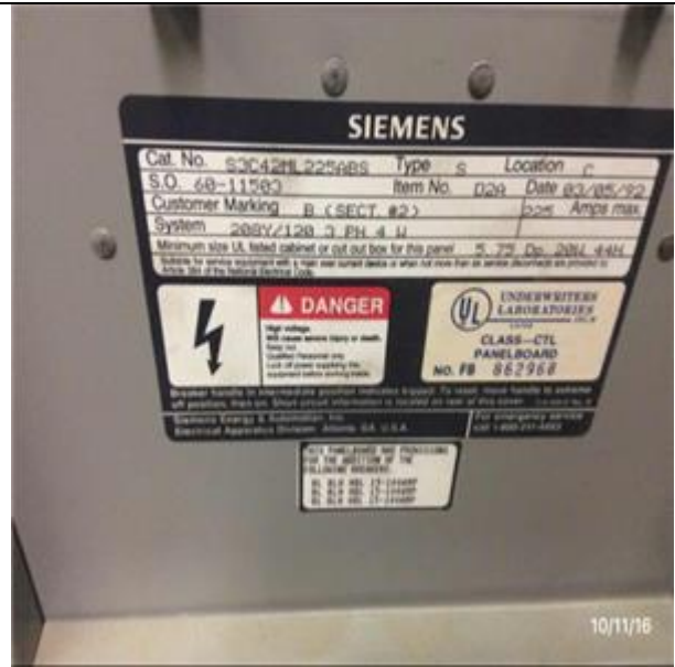
D5012 Low Tension Service & Dist:- View of Panelboard - 120/208volts, 225amp
