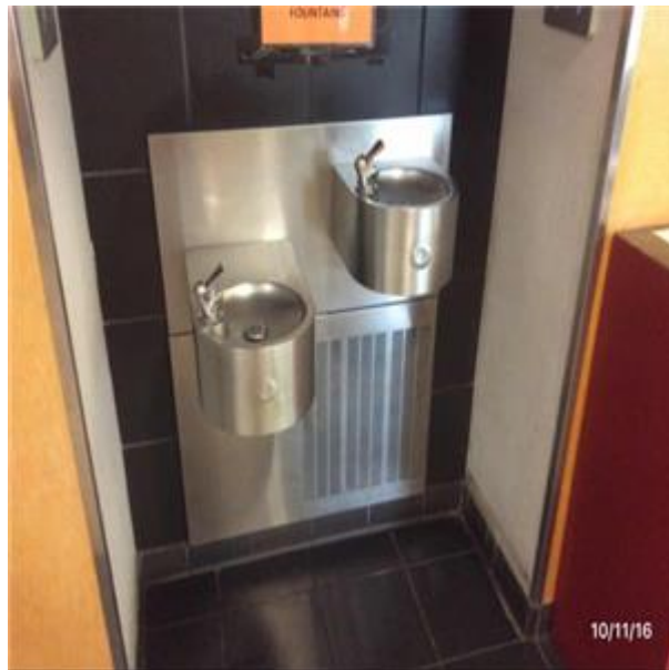
D2018 Drinking Fountains and Coolers:- View of Wall Mounted Standard Drinking Fountain (Single)
