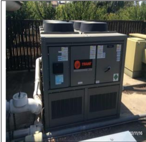
D3052 Package Units:- View of Packaged Outdoor - Cooling Only
