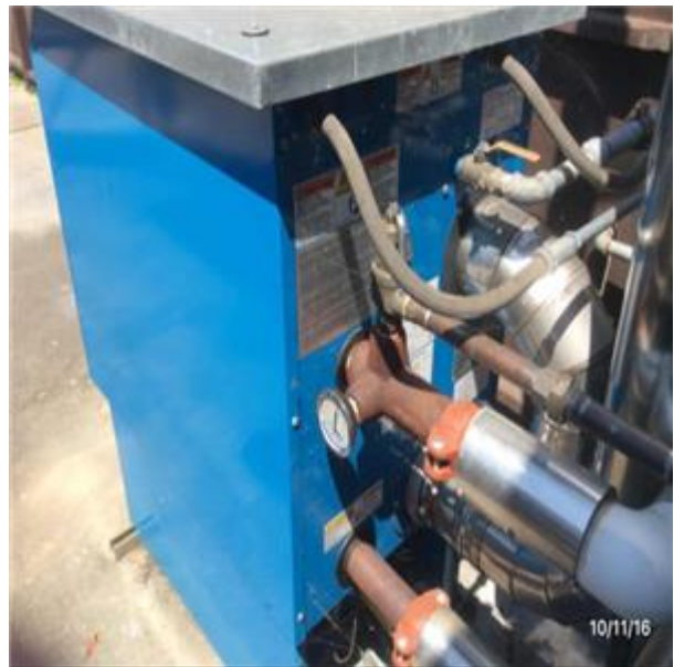
D3021 Boilers:- View of Furnace – Gas
