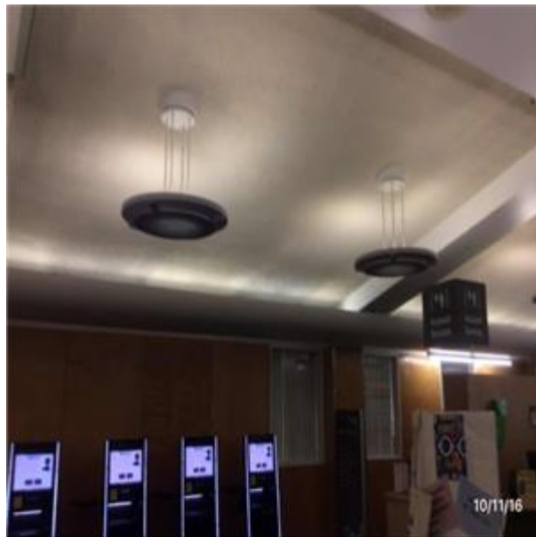
D5022 Lighting Equipment:- View of Feature Light Fixtures to Lobby
