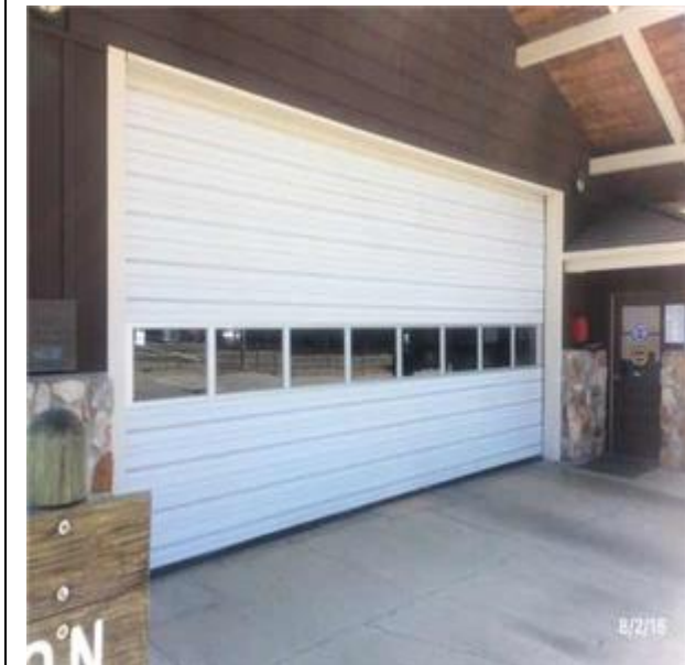
B2034 Overhead Doors:- View of Rolling Overhead Doors, Electric
