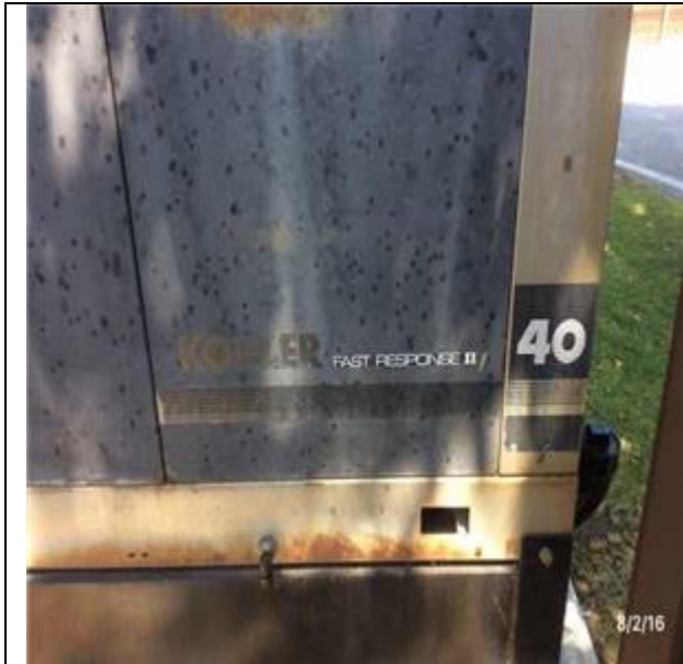
G4092 Site Emergency Power Generation:- View of Generator Sets, Diesel Engine - 50 kW
