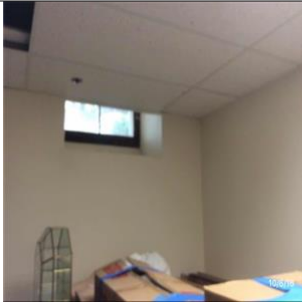
A1011 Wall Foundations:- View of Foundation Wall and Footings up to 12FT - Full Basement
