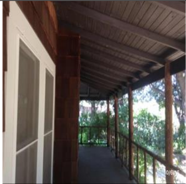
B1023 Canopies:- View of Canopies - Wood Joists Supporting Wood Deck to Porch
