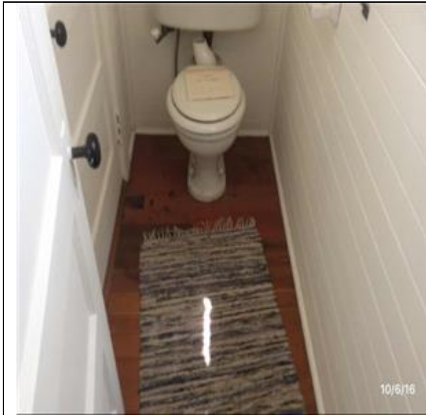
D2011 Water Closets:- View of Floor Mounted Water Closets
