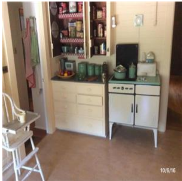
E2012 Fixed Casework:- View of Floor mounted Base Cabinets
