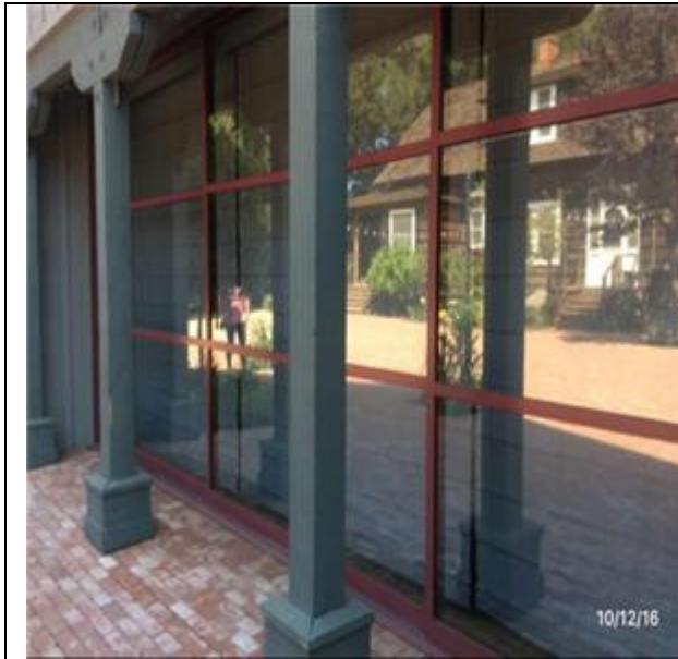
B2031 Glazed Doors & Entrances:- View of Aluminum Glazed Doors - Mall Slider 240 SF
