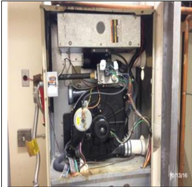
D3021 Boilers:- View of Furnace – Gas
