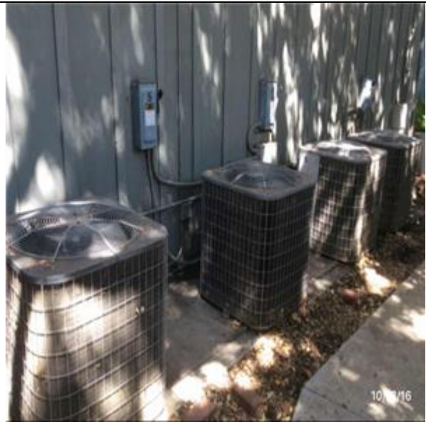
D3032 Direct Expansion Systems:- View of Split-System (Air Cooled Condenser Chiller Unit)
