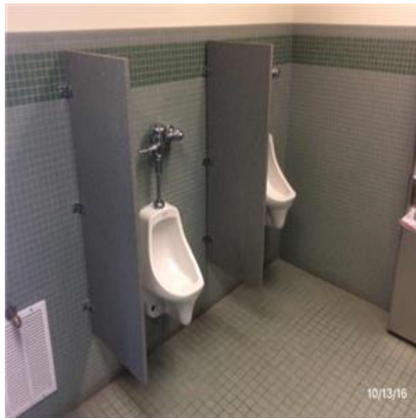
D2012 Urinals:- View of Wall Hung Urinals
