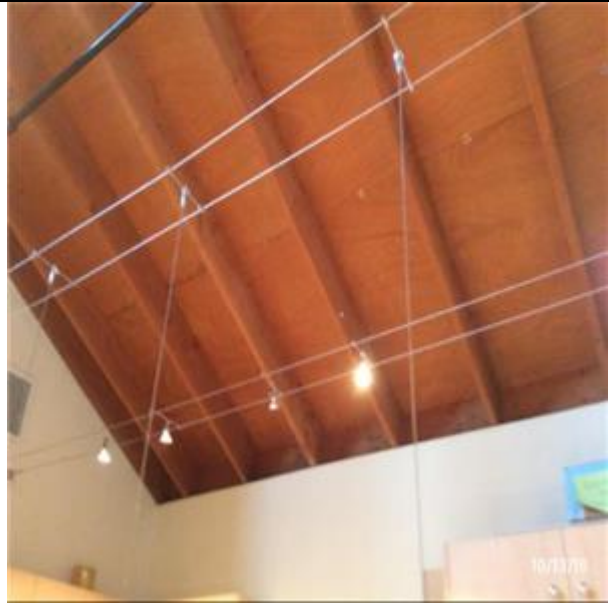
D5022 Lighting Equipment:- View of Interior Light Fixtures - Fluorescent
