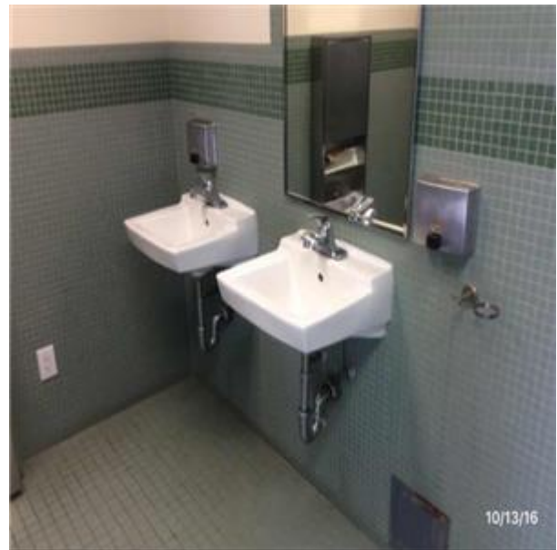
D2013 Lavatories:- View of Wall Hung Lavatories
