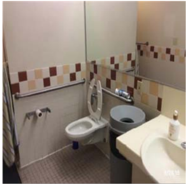
D2011 Water Closets:- View of Wall Mounted Water Closets
