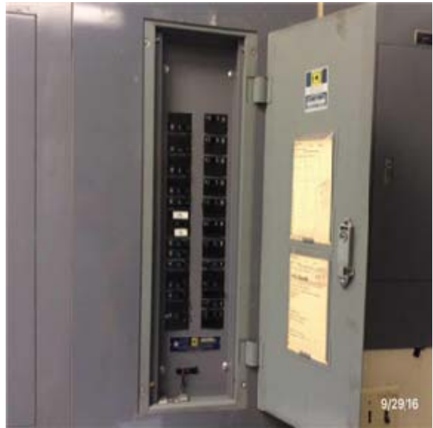
D5012 Low Tension Service & Dist:- View of Panelboard - 120/208volts, 400 to 1200amp
