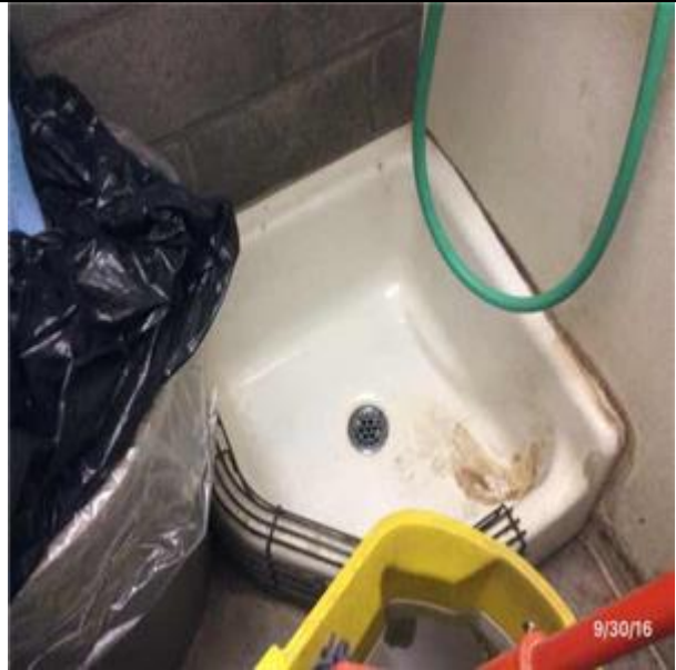
D2014 Sinks:- View of Service Sink Floor Mounted
