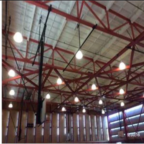
D5022 Lighting Equipment:- View of H.I.D High Bay Fixture(s)
