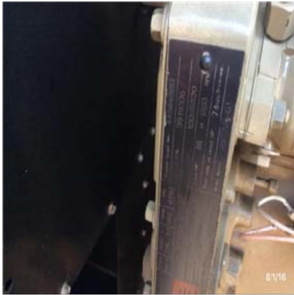
G4092 Site Emergency Power Generation:- View of Generator Sets, Diesel Engine - 50 kW
