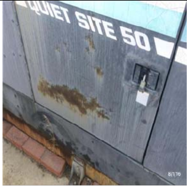
G4092 Site Emergency Power Generation:- View of Generator Sets, Diesel Engine - 50 kW
