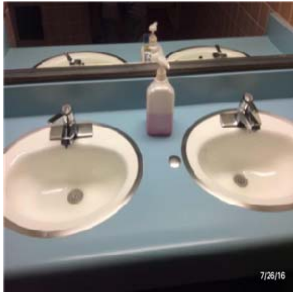
D2013 Lavatories:- View of Vanity Top Lavatories
