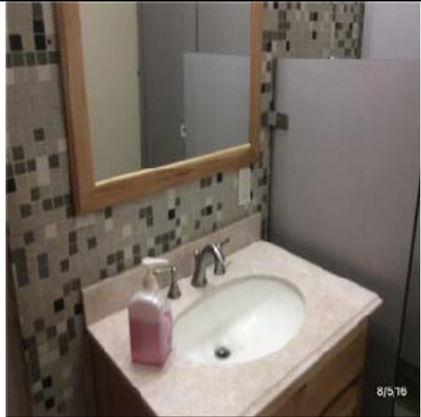
D2013 Lavatories:- View of Vanity Top Lavatories
