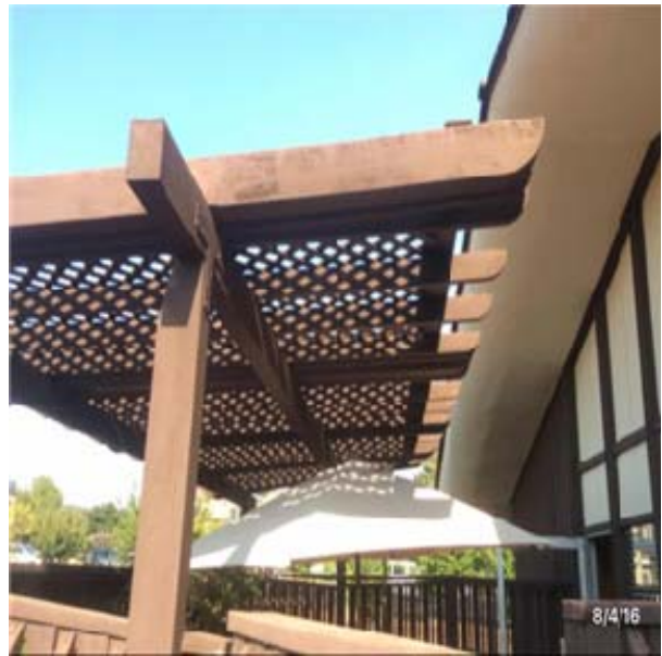
B2014 Exterior Sun Control Devices:- View of Exterior Sun Control Devices
