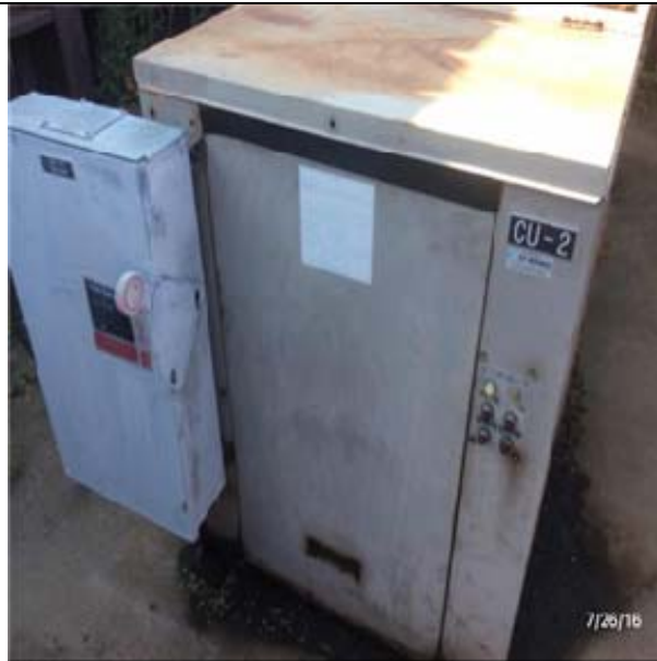
D3032 Direct Expansion Systems:- View of Split-System (Air Cooled Condenser Chiller Unit)
