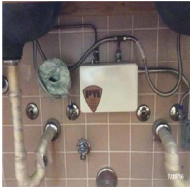
D2022 Hot Water Service:- View of insta-hot under counter water heater (no storage tank)
