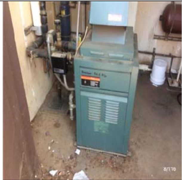
D3021 Boilers:- View of HW Boiler - Oil/Gas - 205 to 1000 MBH Range
