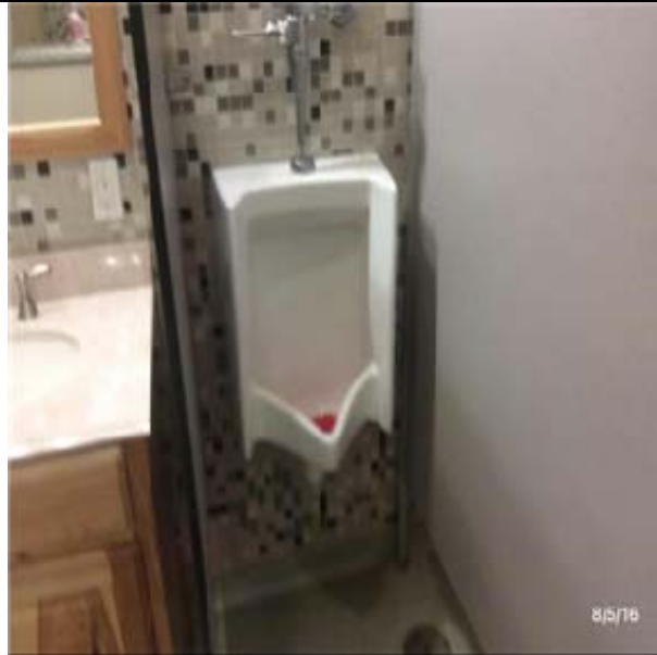
D2012 Urinals:- View of Wall Hung Urinals
