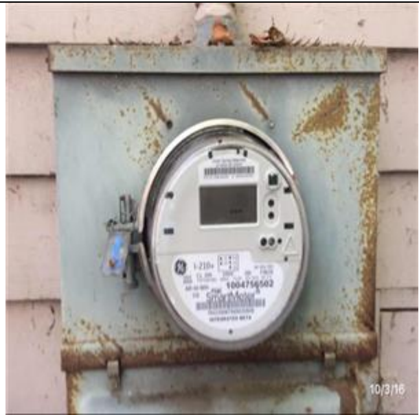
D5012 Low Tension Service & Dist:- View of Panelboard - 120/240volts, 60 to 2000amp
