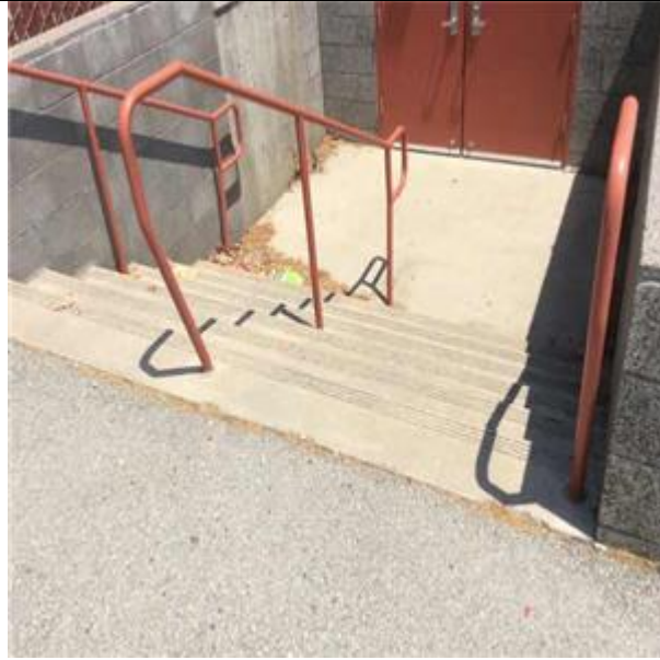
B1015 Exterior Stairs and Fire Escapes:- View of Exterior Stair(s) - Concrete Construction
