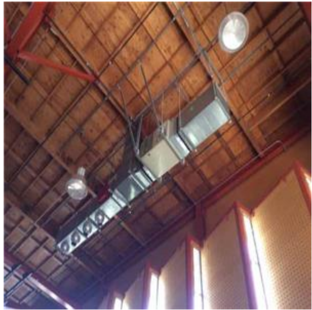
D3021 Boilers:- View of Furnace – Gas
