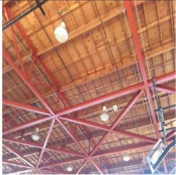
B1021 Flat Roof Construction:- View of Roof Construction - Structural Steel Beams and Joist with Timber Roof Deck
