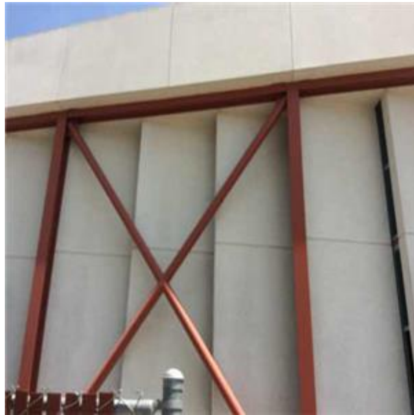
B1031 Steel Frame Structure:- View of Structural Steel Columns and Beams Frame
