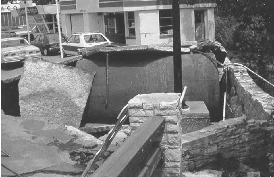
Figure 3.2.3.1A: Tank lifted by buoyancy forces
