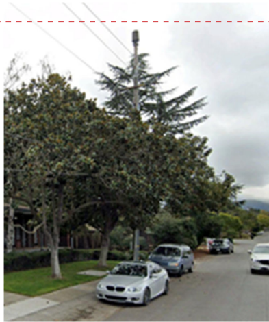
Figure 7: Landscaping conceals wireless telecommunications equipment mounted on the exterior of this pole located on Distel Drive.
