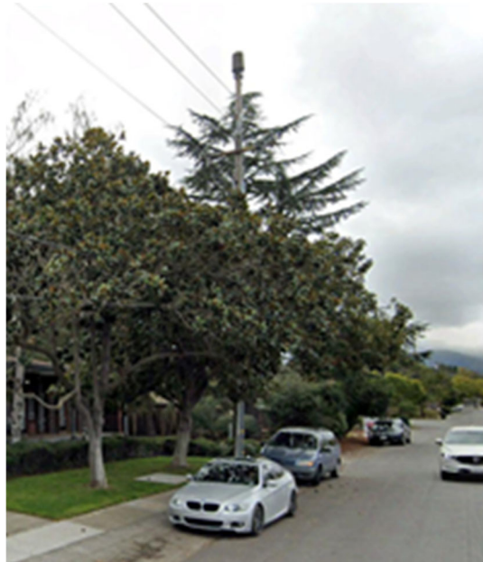
Figure7: Landscaping conceals wireless telecommunications equipment mounted on the exterior of this pole located on Distel Drive.
