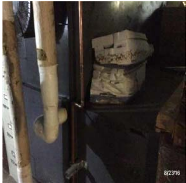
D3041 Air Distribution Systems:- View of AHU - Constant Volume #2
