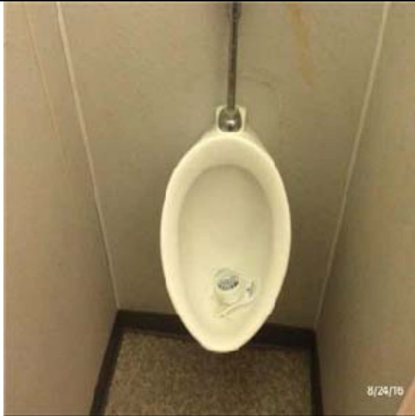
D2012 Urinals:- View of Wall Hung Urinals
