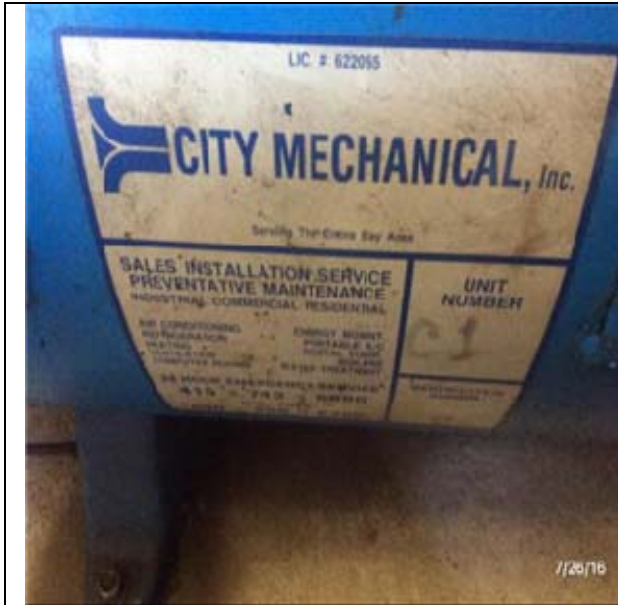
D2099 Other Piping Systems:- View of Air Compressor - 2 H.P.
