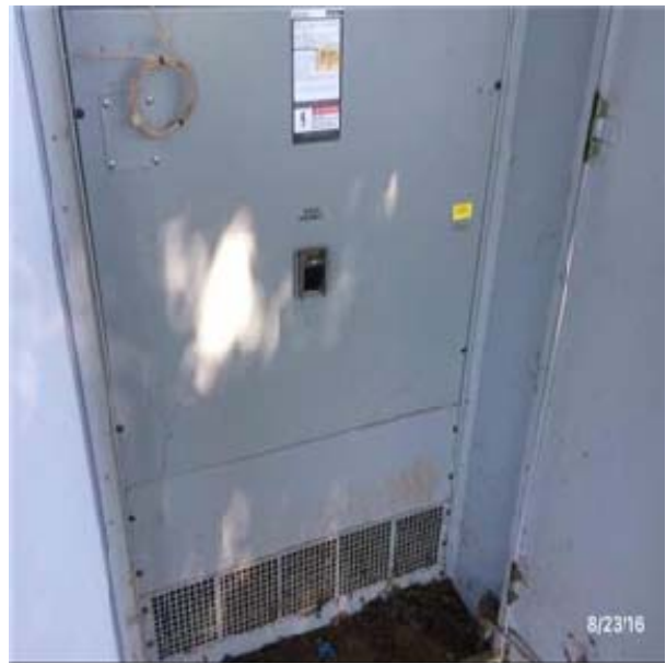
D5012 Low Tension Service & Dist:- View of Panelboard - 120/208volt, 60 to 2000amp
