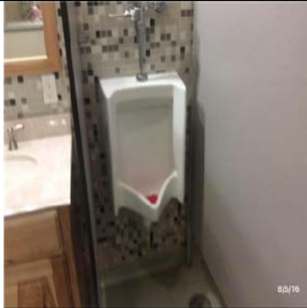
D2012 Urinals:- View of Wall Hung Urinals
