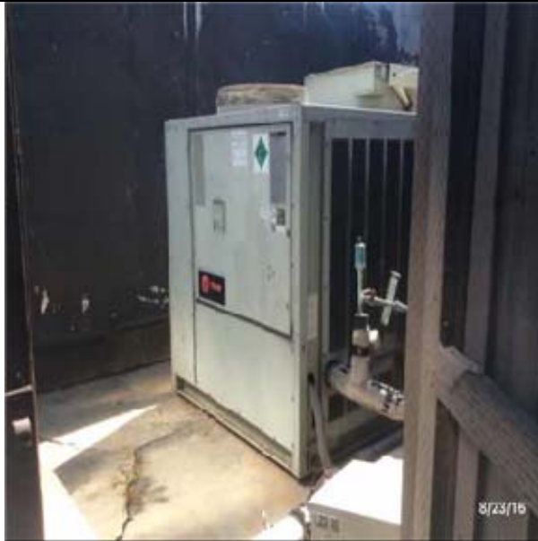
D3031 Chilled Water Systems:- View of Air Cooled Water Chiller Unit - Outdoor Unit
