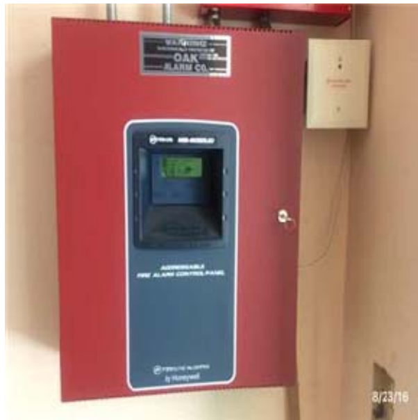
D5037 Fire Alarm Systems:- View of Fire Alarm Control Panel (FACP) - Up to 10 Zone
