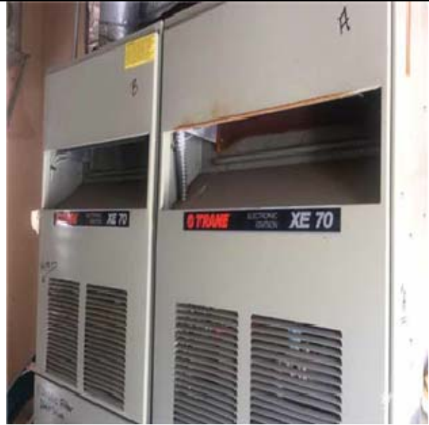
D3032 Direct Expansion Systems:- View of Split-System (Indoor Furnace Unit) 101 to 150 BTU
