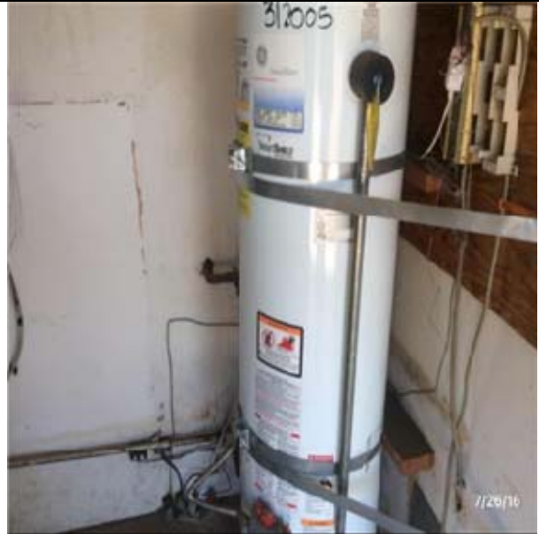
D2022 Hot Water Service:- View of Domestic Hot Water Heater - Gas
