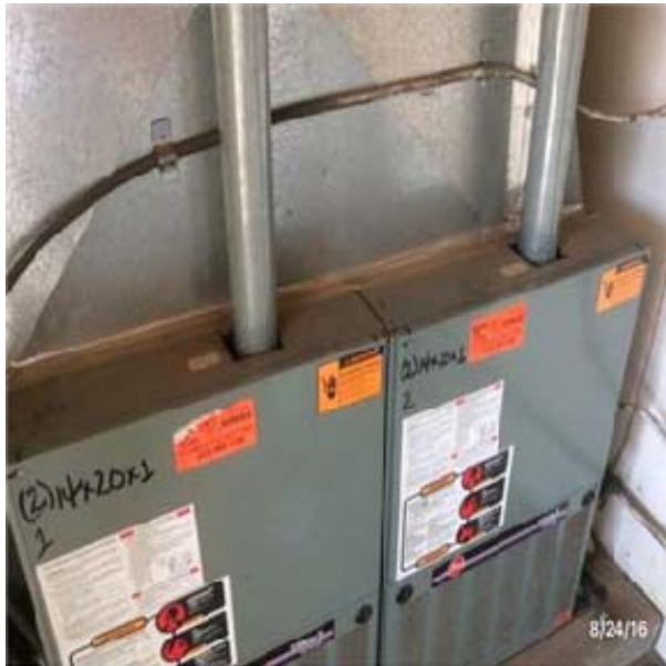
D3021 Boilers:- View of Furnace - Gas #1
