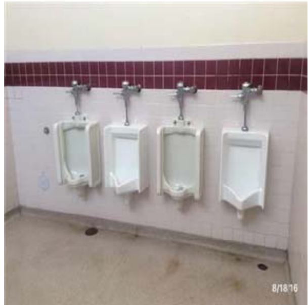
D2012 Urinals:- View of Wall Hung Urinals
