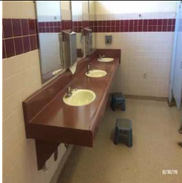
D2013 Lavatories:- View of Vanity Top Lavatories
