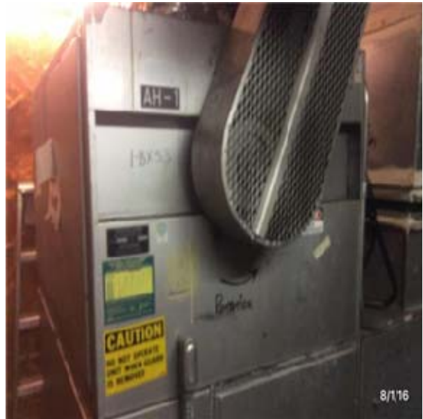
D3041 Air Distribution Systems:- View of AHU - VAV System
