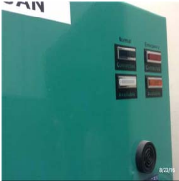
D5012 Low Tension Service & Dist:- View of Emergency Transfer Switch
