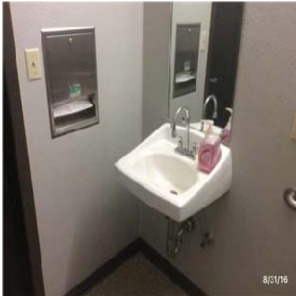
D2013 Lavatories:- View of Wall Hung Lavatories
