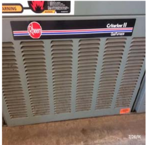
D3021 Boilers:- View of Furnace - Gas #2
