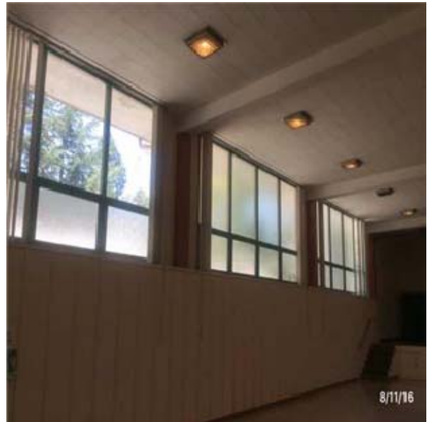
D5022 Lighting Equipment:- View of H.P. Sodium Fixtures
