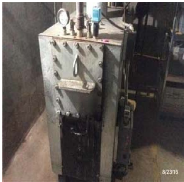
D3021 Boilers:- View of Domestic Hot Water Boiler – Gas
