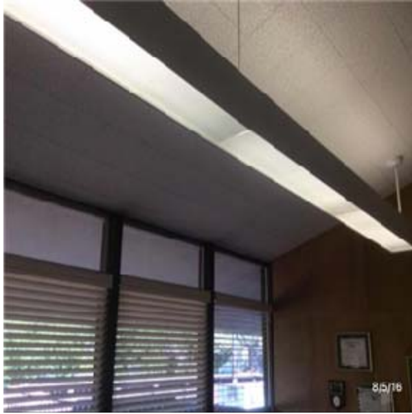
D5022 Lighting Equipment:- View of Z_LEGACY Fluorescent Strip Light Fixtures
