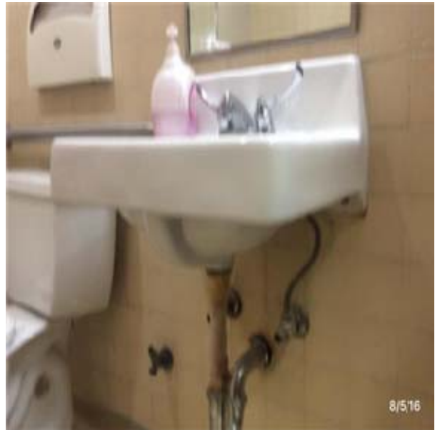
D2013 Lavatories:- View of Wall Hung Lavatories
