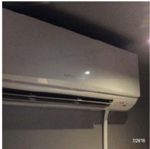
D3032 Direct Expansion Systems:- View of Split-System (Indoor Unit Only - Cooling, Heating Coils and Circulation Fan)
