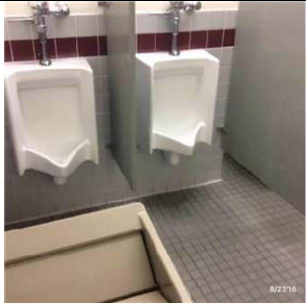
D2012 Urinals:- View of Wall Hung Urinals
