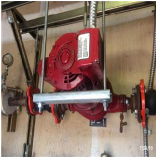
D3022 Boiler Room Piping & Specialties:- View of Boiler Circulation Pump/Motors 1 H.P.
