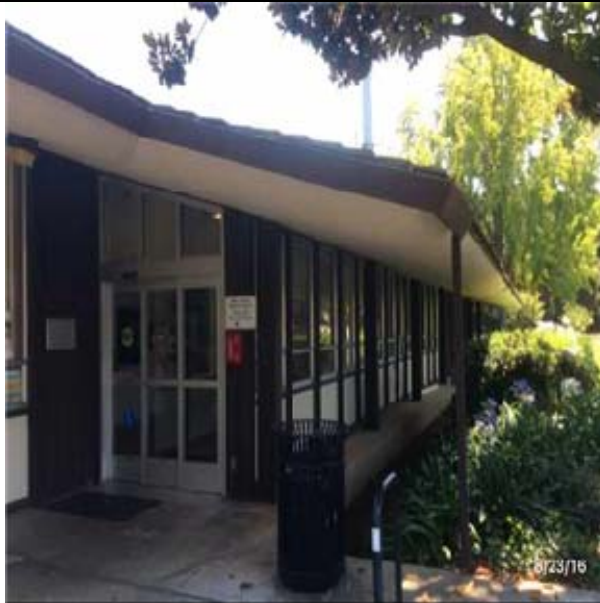
D5022 Lighting Equipment:- View of Exterior Wall Pack Light Fixtures
