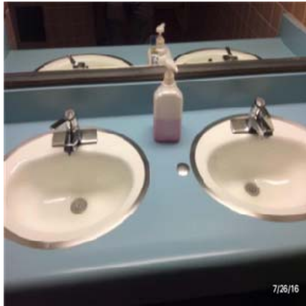
D2013 Lavatories:- View of Vanity Top Lavatories
