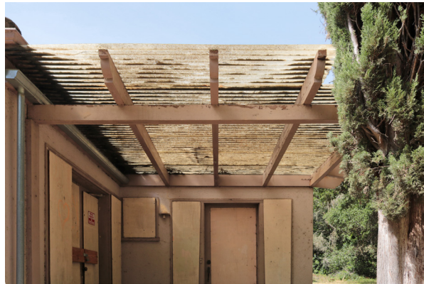
Corrugated plastic roof at pergola (ARG, 2019).
