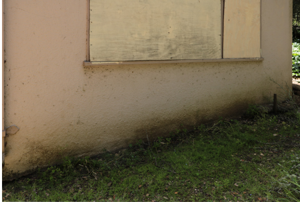
Biological growth along base of exterior wall at east elevation (ARG, 2019).
