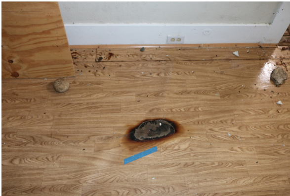
Burn damage at the floor of the Animal Room (ARG, 2019).
