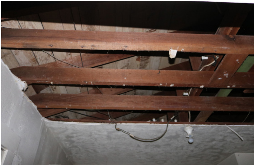
View of exposed framing where west wing kitchen ceiling has partially collapsed.
