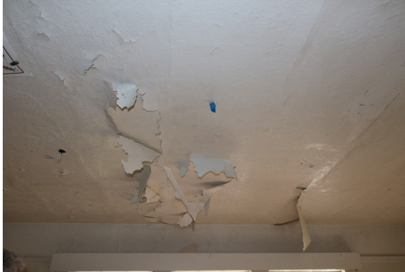
Delamination of plaster at the Discovery Lab (ARG, 2019).
