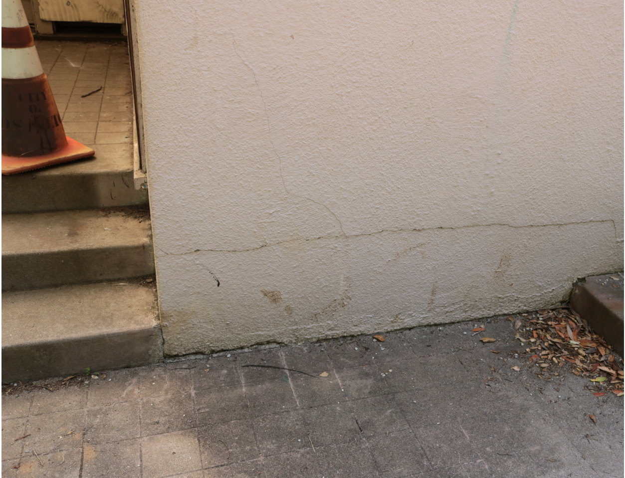
Existing stucco conditions at north elevation adjacent to main entrance.
