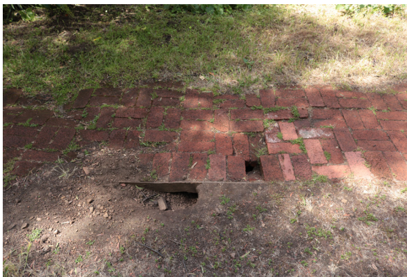
Detail view of brick path at east side of building. Note the soil erosion and uneven surface (ARG, 2019).
