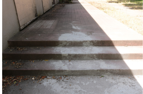
Paint stain at the north terrace stairs (ARG, 2019).
