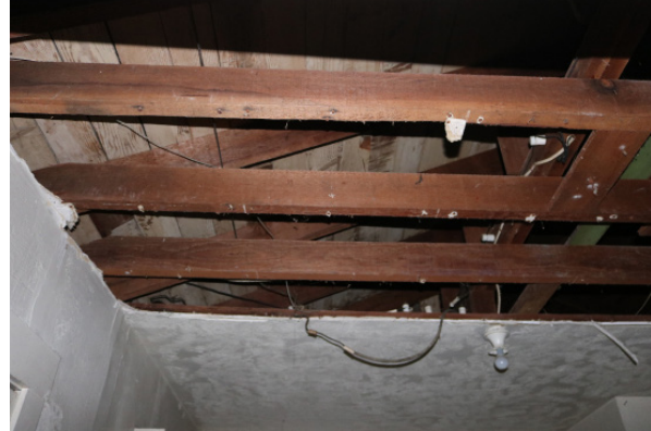
Missing drywall in the East Kitchen (ARG, 2019).
