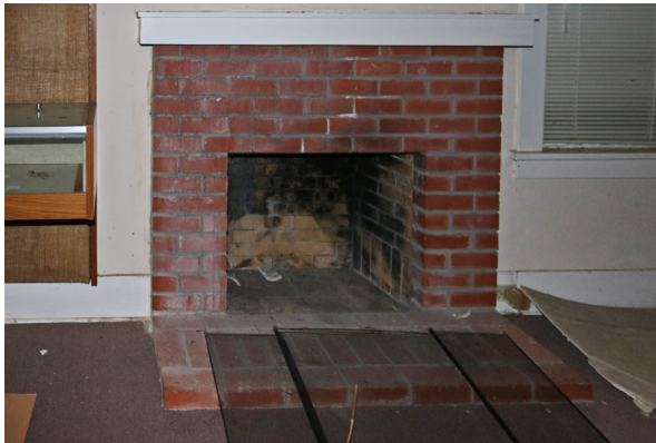
Fireplace in the Ohlone Room. Note the soot damage at the firebox (ARG, 2019).
