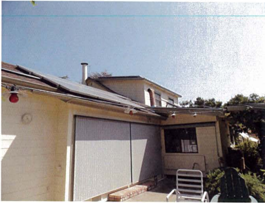
Figure 14. South elevation with Pool Room addition to the left and enclosed porch/kitchen addition to the right with overhang (Garavaglia Architecture, Inc., August 2015)
