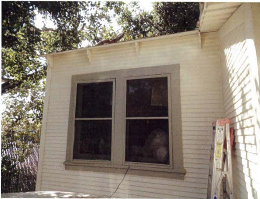
Figure 26. Western portion of Garage north elevation, likely original windows and roofline brackets (Garavaglia Architecture, Inc., August 2015)
