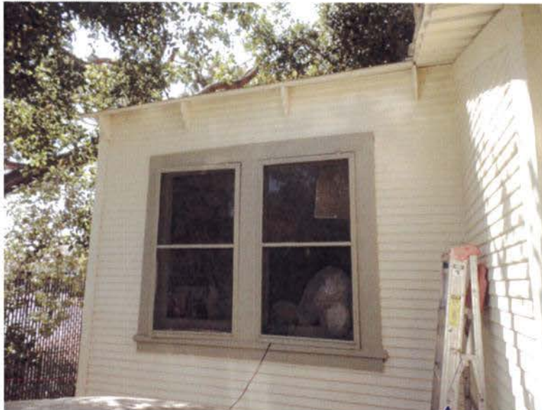
Figure 12. Western portion of Garage north elevation, likely original windows and roofline brackets (Garavaglia Architecture, Inc., August 2015)
