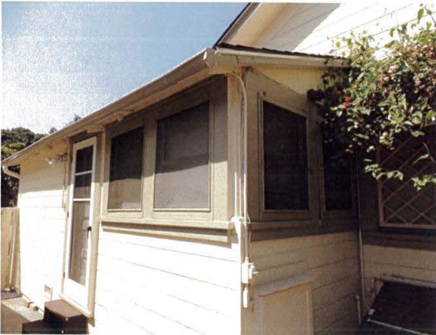
Figure 12. Detail of side addition at eastern elevation. Note the difference in siding material and window at right (Garavaglia Architecture, Inc., August 2015)
