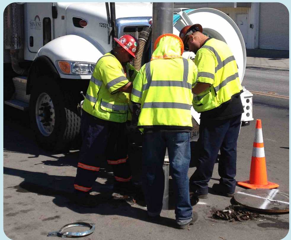
▲ Member agency staff work together to maintain the storm drain system.
