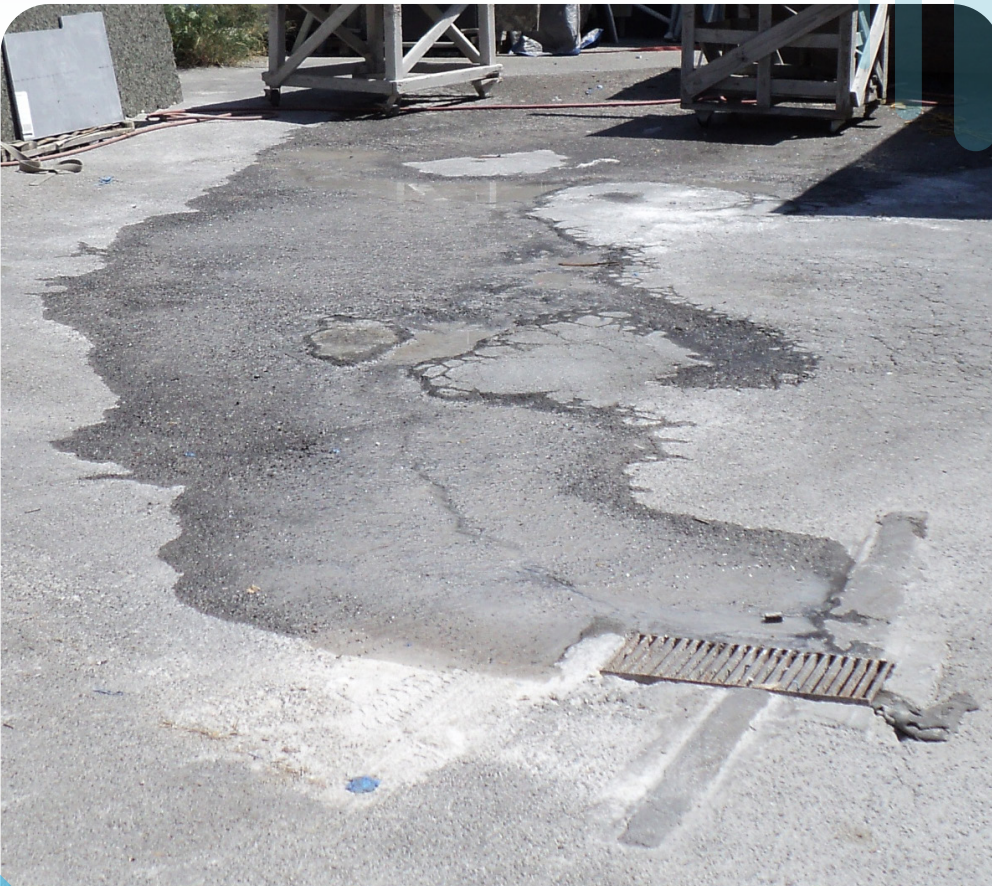
▼ Illicit discharge flowing into storm drain
