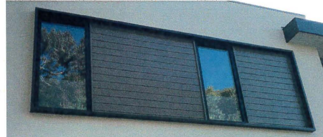
STAINED WOOD BETWEEN WINDOWS
