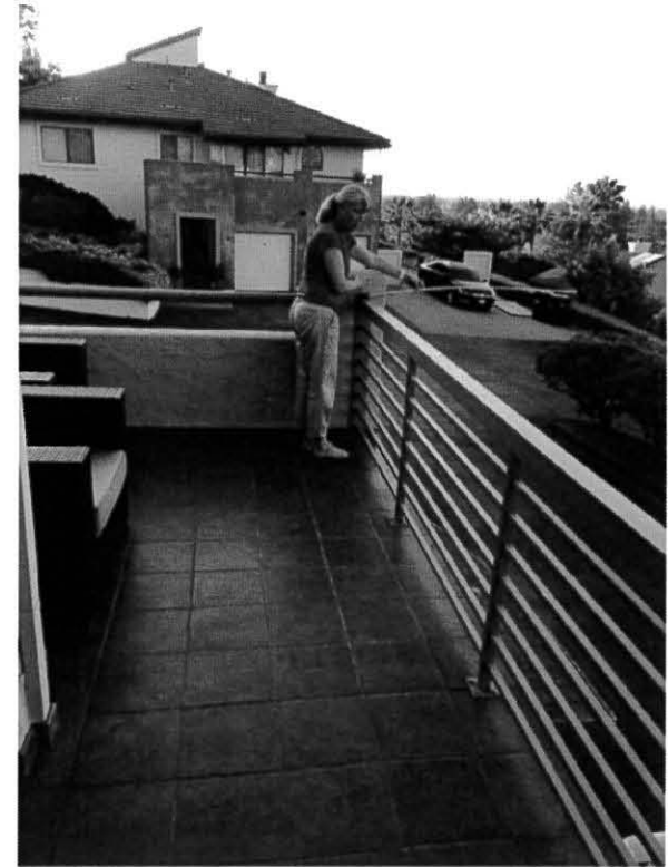
THE DECK WILL BE EXTENDED TO THE END OF THE MEASURING TAPE AS SHOWN IN THE PHOTO ABOVE.
