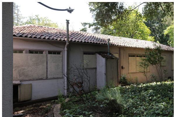
Plant growth along west elevation (ARG, 2019).
