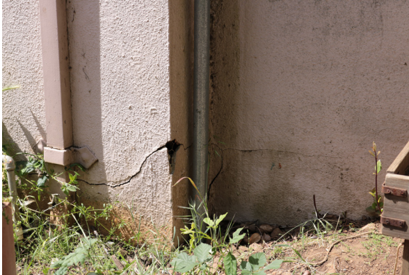
Major stucco spall at the base of the northeast corner (ARG, 2019).
