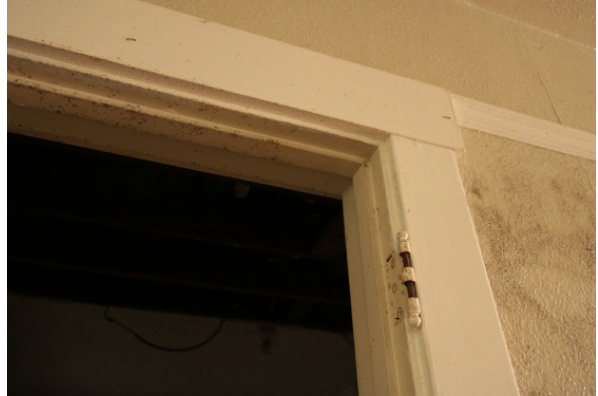
Mold along the wall and door trim at the north wall of the West Kitchen (ARG, 2019).
