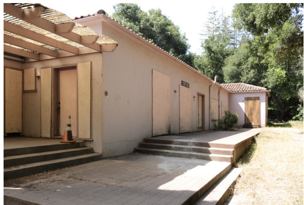
View of north elevation looking west. Note the lack of handrails at both sets of stairs (ARG, 2019).
