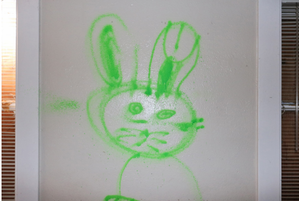
Graffiti on the east wall of the Animal Room (ARG, 2019).
