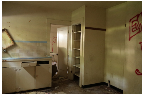
Note the missing door at the pantry of the West Kitchen (ARG, 2019).
