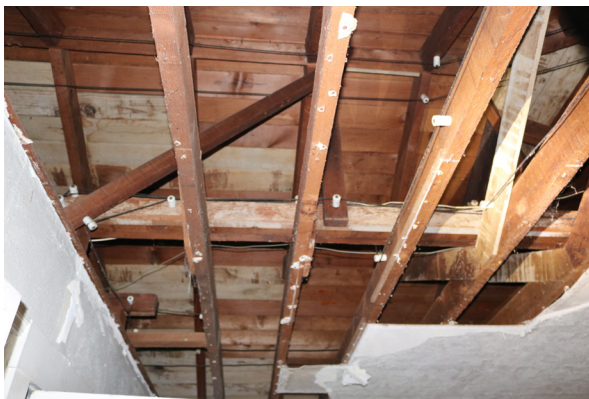
Missing drywall in the Craft Room (ARG, 2019).
