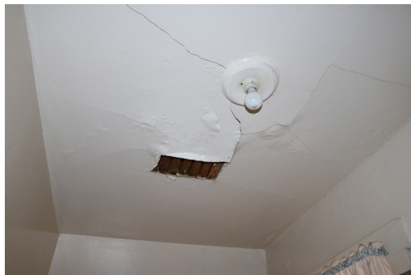
Water damage and exposed lath in East Restroom (ARG, 2019).
