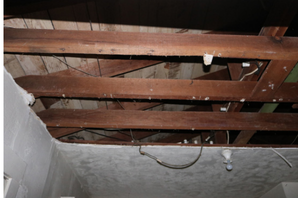
Missing drywall in the East Kitchen (ARG, 2019).
