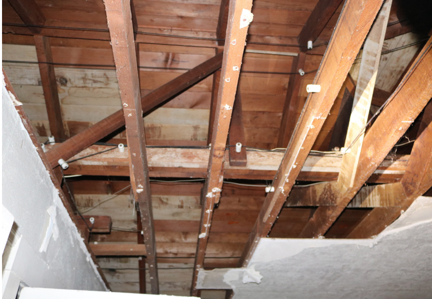
Craft room, view of partially collapsed ceiling and exposed roof framing.
