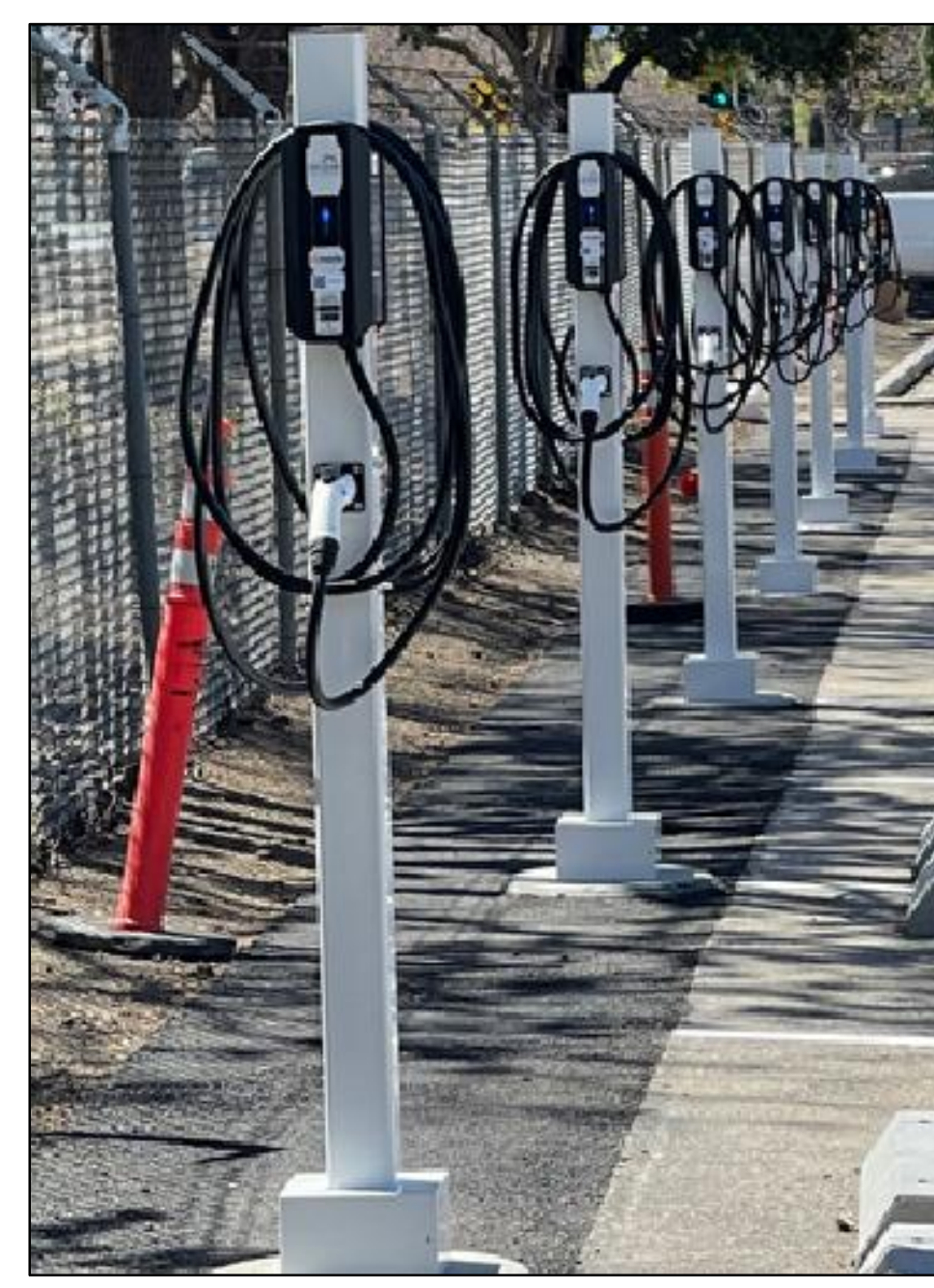
EV CHARGER FREE STANDING PORT
