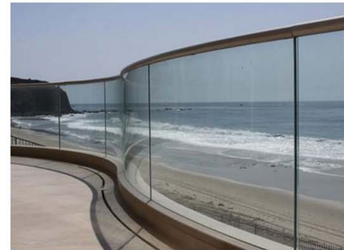
DECK MOUNTED GLASS GAURD RAILINGS
