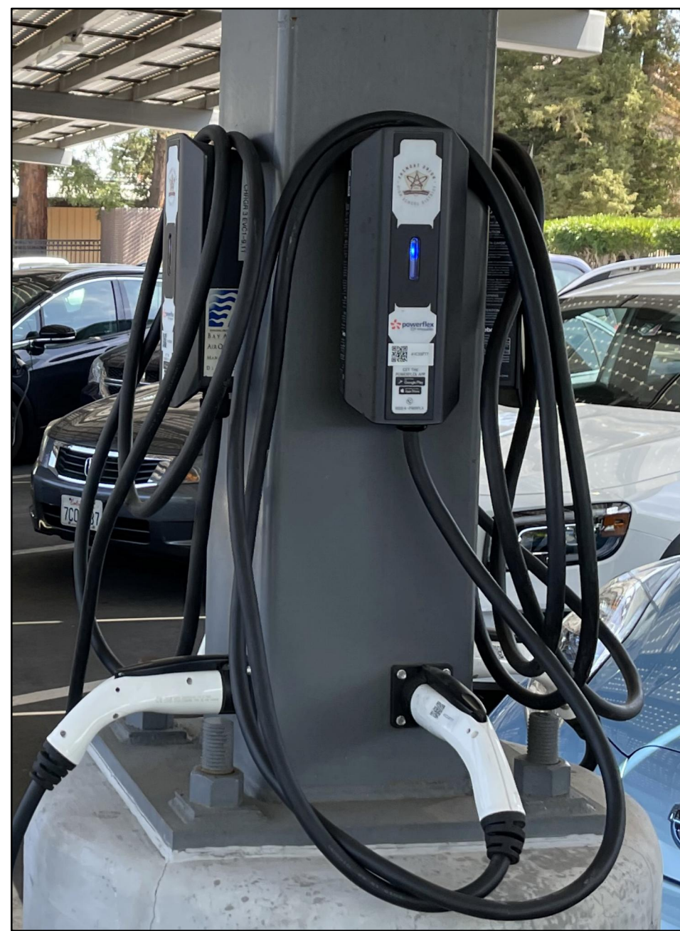
EV CHARGER COLUMN MOUNTED
