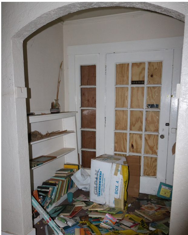
View inside niche at east wall of main room, looking east toward entry.
