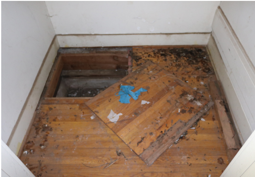
View of access panel at floor inside closet at south end of east wing.
