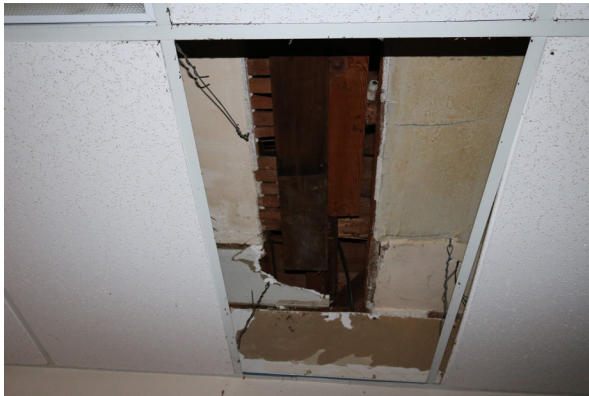
Missing section of acoustic tile with underlying damaged plaster and lath in the Main Room (ARG, 2019).
