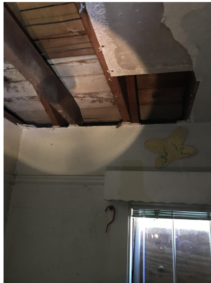
Photo #14: Roof Framing and Ceiling Joist at East Wing of the Building
