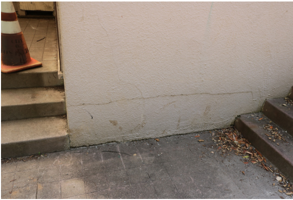
Crack along the base of the north elevation at the Main Entry (ARG, 2019).
