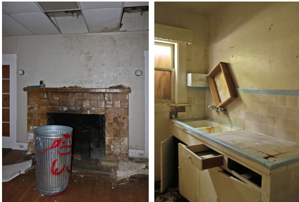
Water damage above fireplace in the Main Room (left); damaged casework and tile of the West Kitchen (right); (ARG, 2019).
