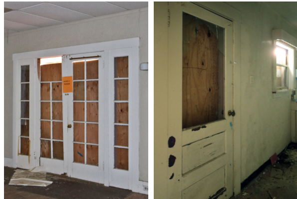
Typical original French doors in the Main Room (left); damaged exterior door at the East Kitchen (right); (ARG, 2019).
