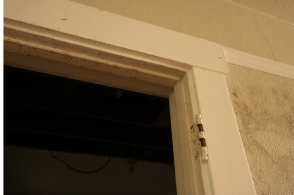
Mold along the wall and door trim at the north wall of the West Kitchen (ARG, 2019).
