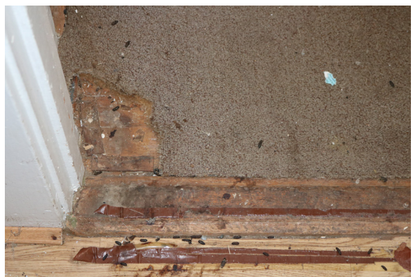
Section of missing carpet revealing the original wood flooring beneath in the West Hall (ARG, 2019).
