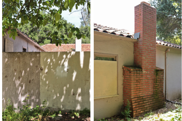
Dissimilar paint colors along the south elevation (left); biological growth at the west chimney (right); (ARG, 2019).
