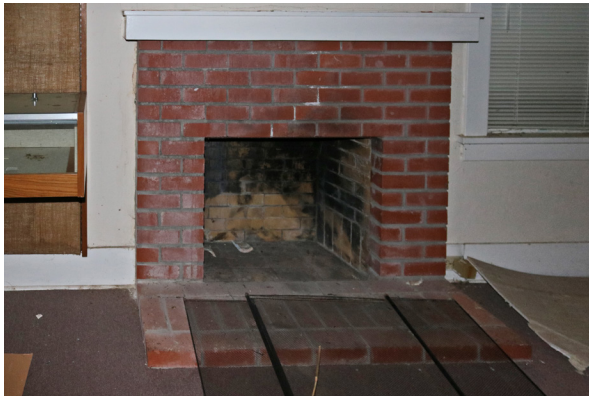
Fireplace in the Ohlone Room. Note the soot damage at the firebox (ARG, 2019).
