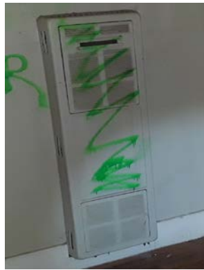
M2.2 Wall Heater
