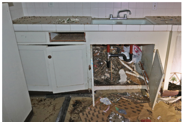
Large rodent nest at the sink base cabinet in the East Kitchen. Note the missing drawer and missing hardware (ARG, 2019).
