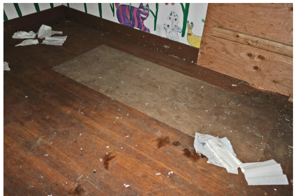
Plywood patch at the wood floor in the Kid's Room (ARG, 2019).
