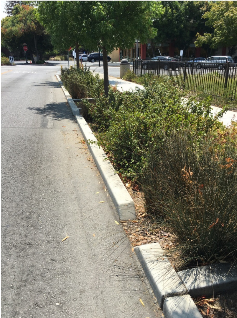
Figure 2- Example Rain Garden on 2nd Street, Los Altos (NCE)
