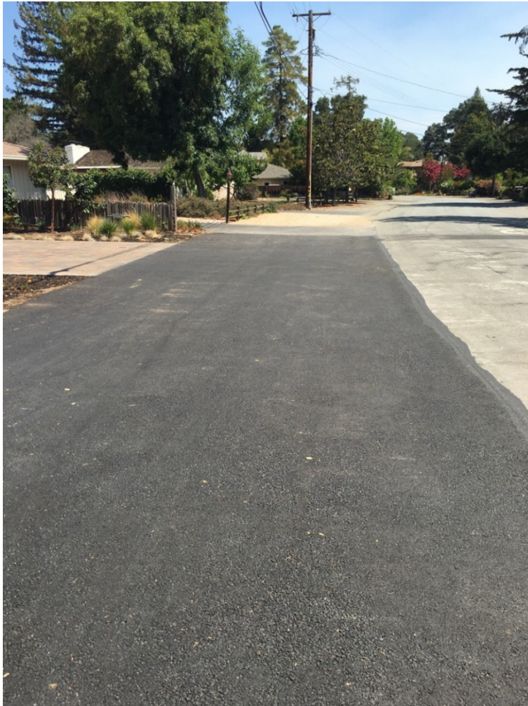
Figure 1 - Asphalt used in shoulder parking and drainage swale area (NCE)
