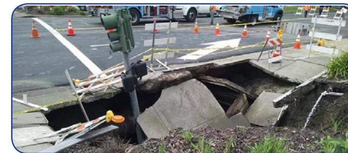
A 30 foot by 15 foot deep sinkhole on Rheem Blvd that developed due to a broken drain pipe on March 13, 2016.
