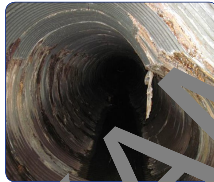
A broken drainage pipe can lead to another major sink hole. (SDMP)
