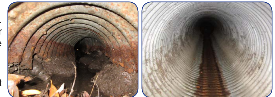
A drainage pipe with the bottom rusted away in comparison to an intact drainage pipe (2015 SDMP)
