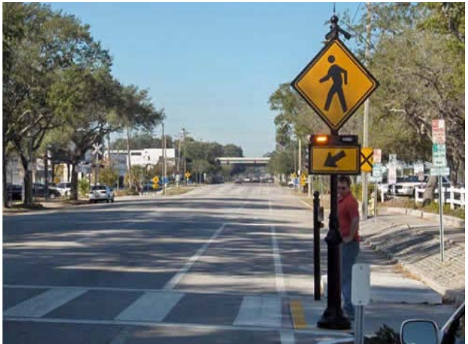
Rectangular Rapid Flashing Beacon
